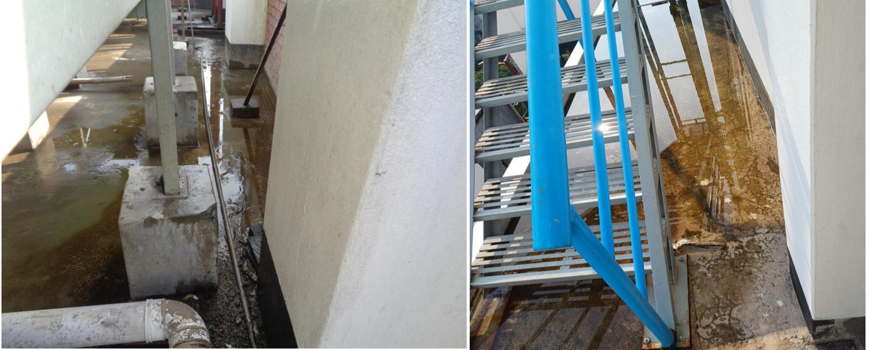
Water ponding on roof
