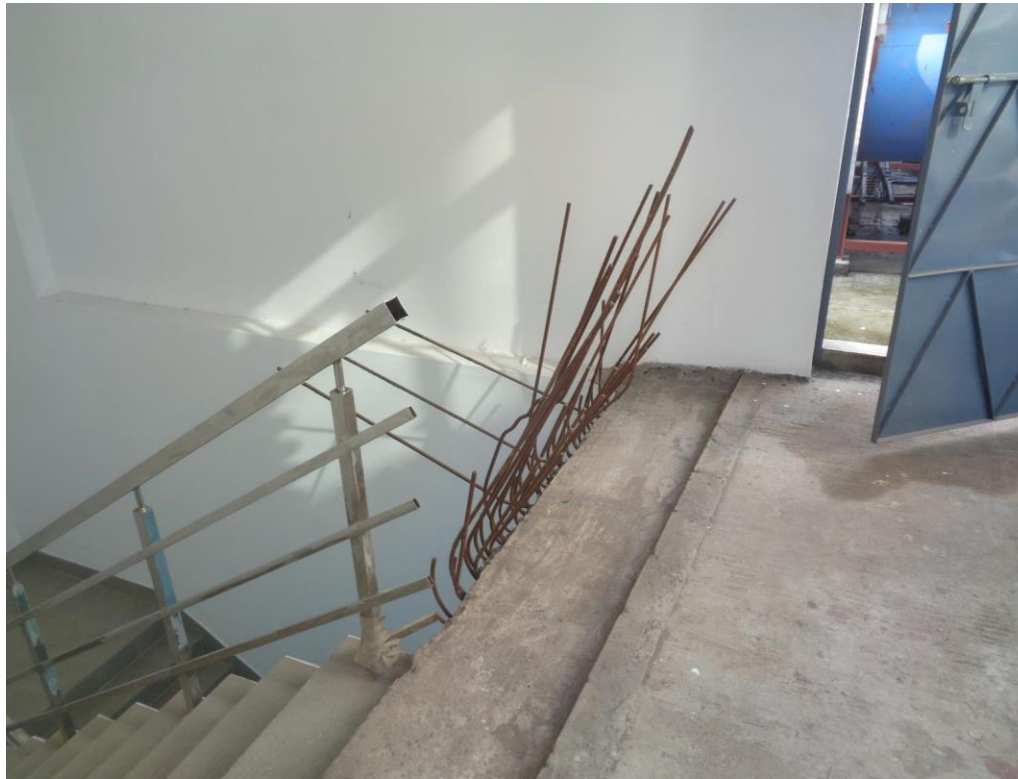
Exposed rebar and falling hazard in stair
