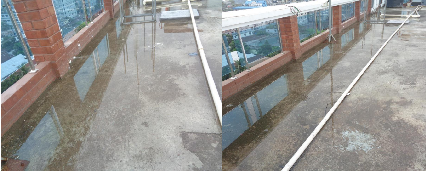
Water ponding on roof
