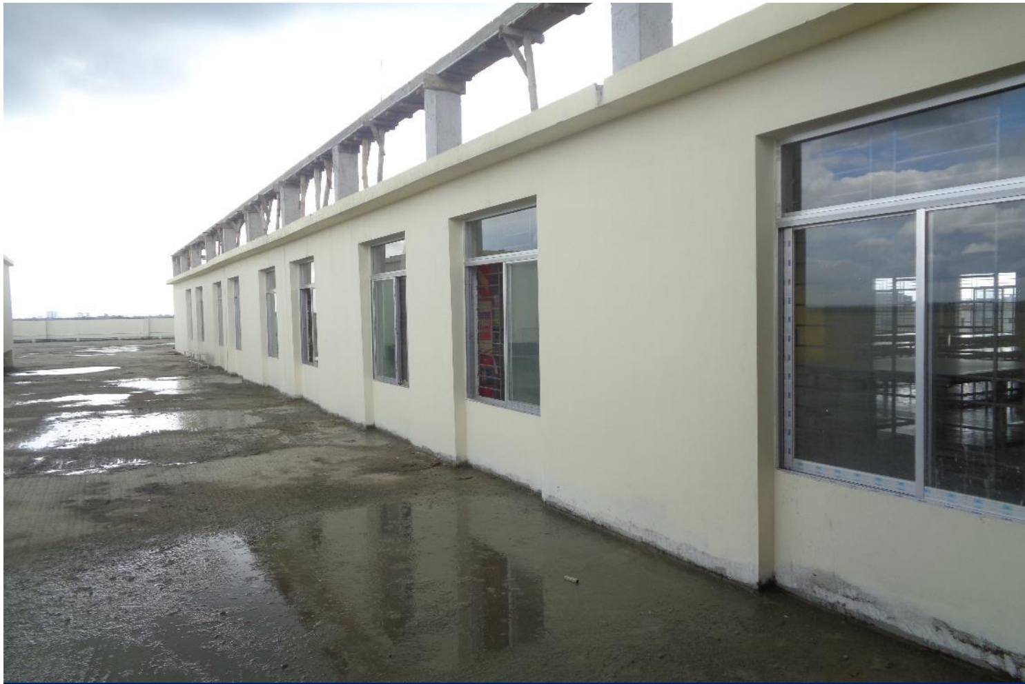
Water ponding observed on roof slab
