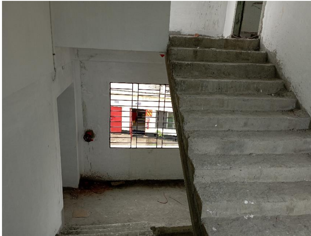
Railing was missing at staircase
