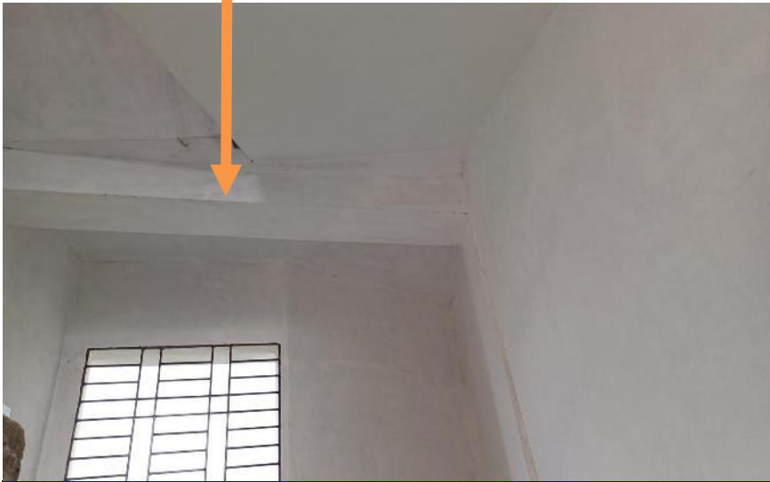
No diagonal but straight beam at stair
