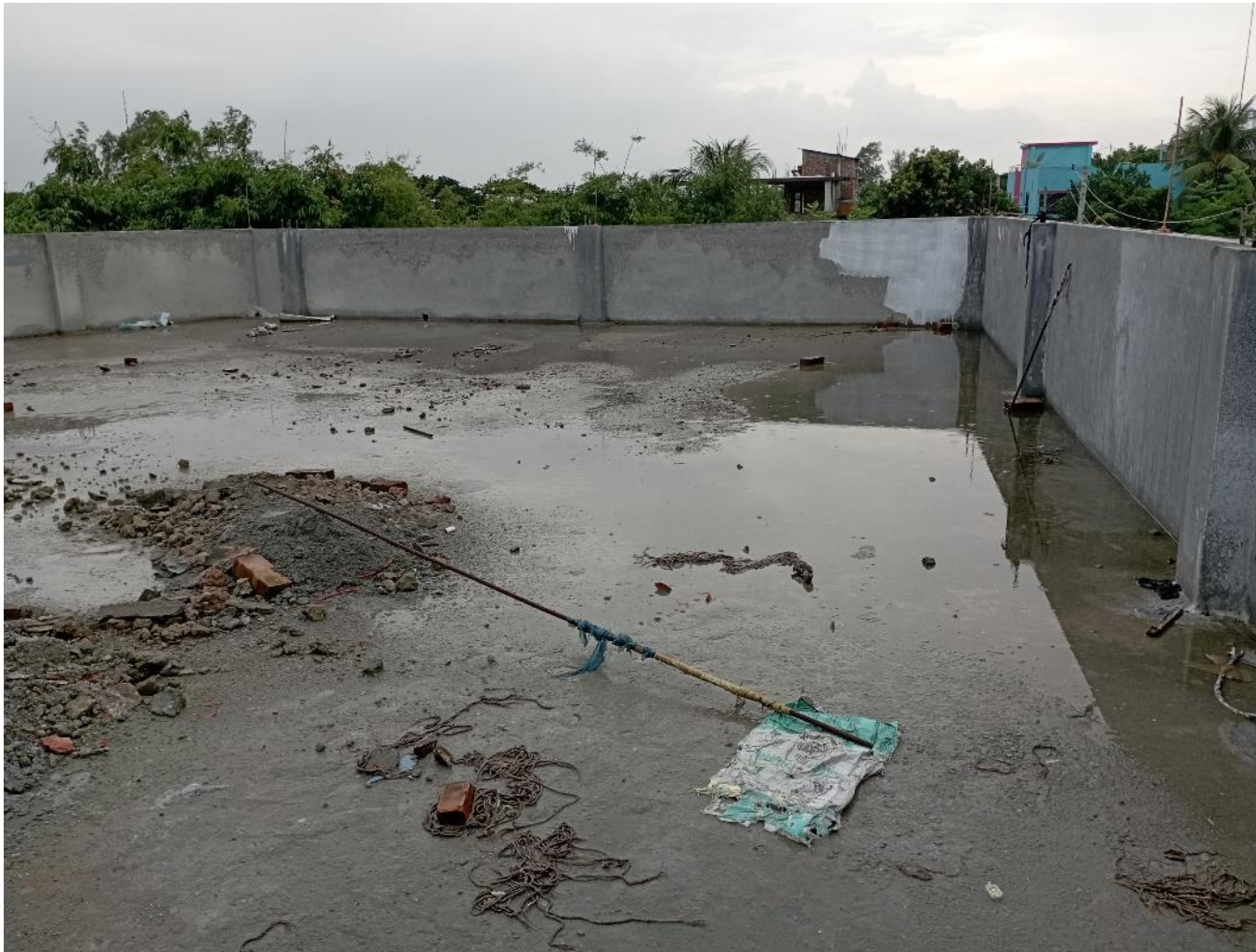
Water ponding observed on roof slab
