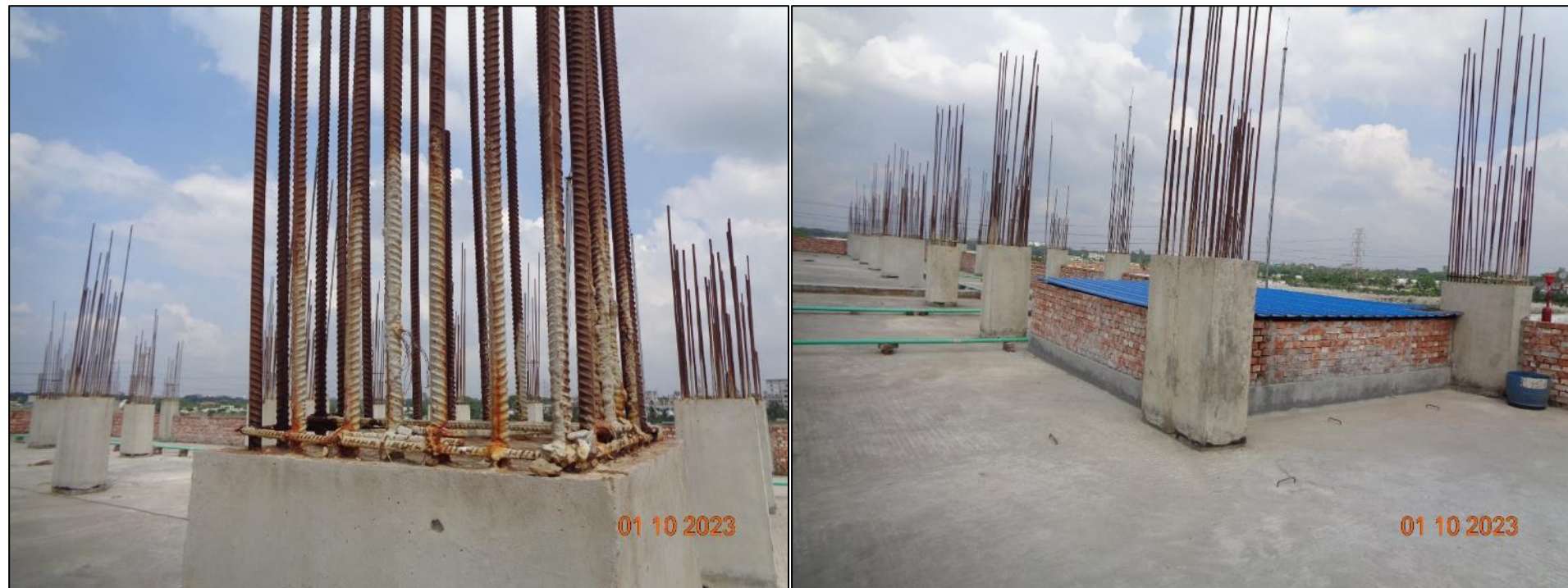
Exposed rebar of Column
