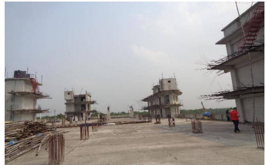
Projected rebar observed at roof level
