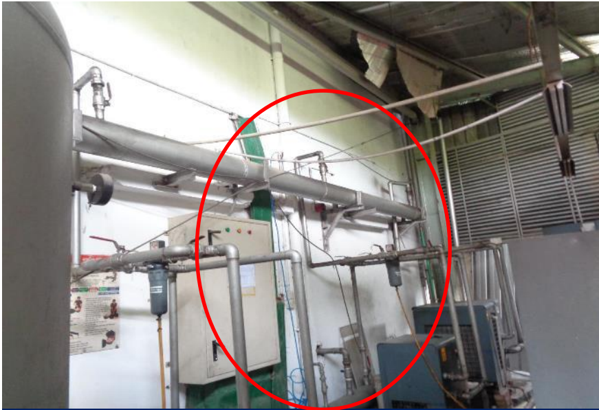
Torn cable bracing (Compressor Shed)
