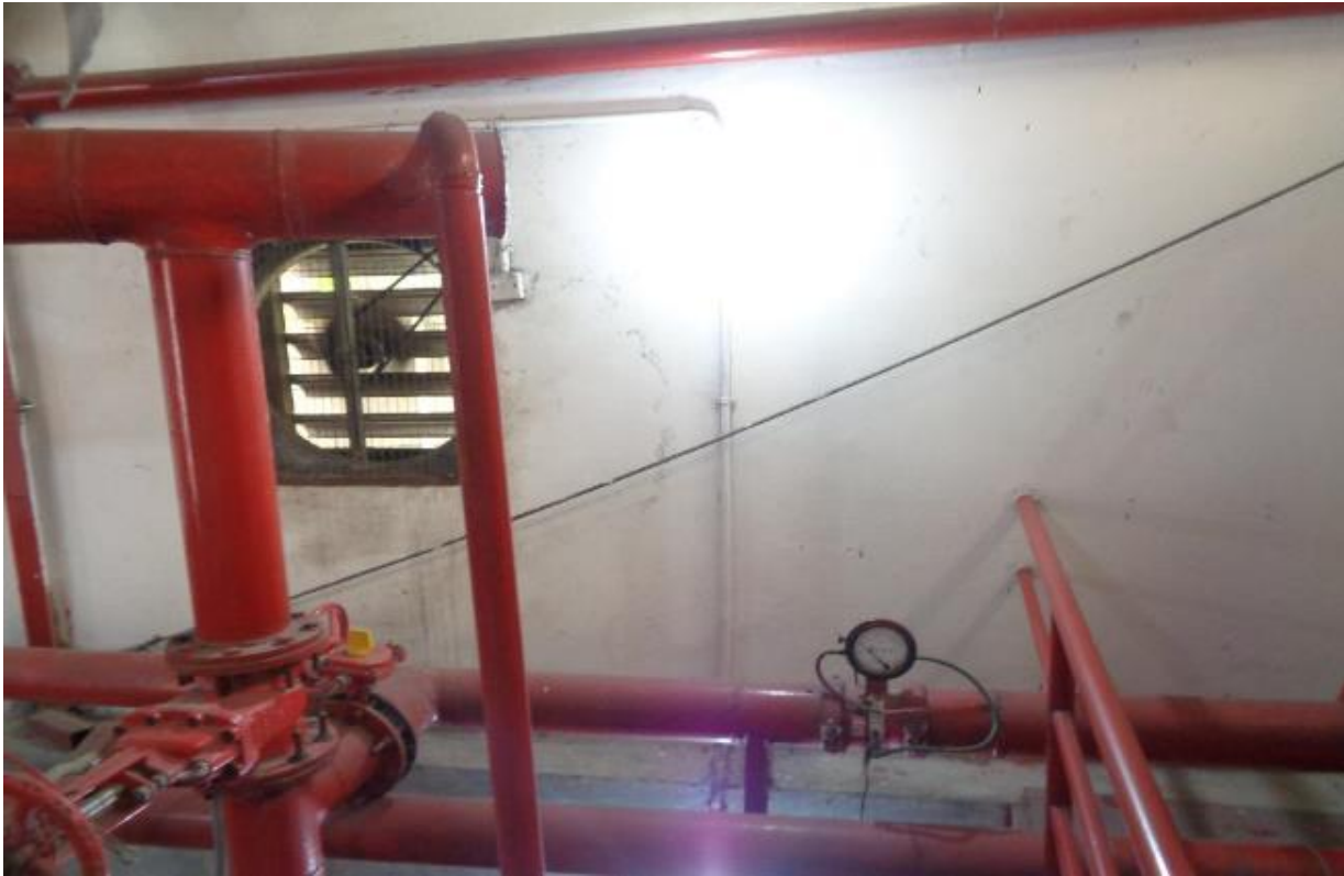
Loose cable bracing (Fire Pump Shed)
