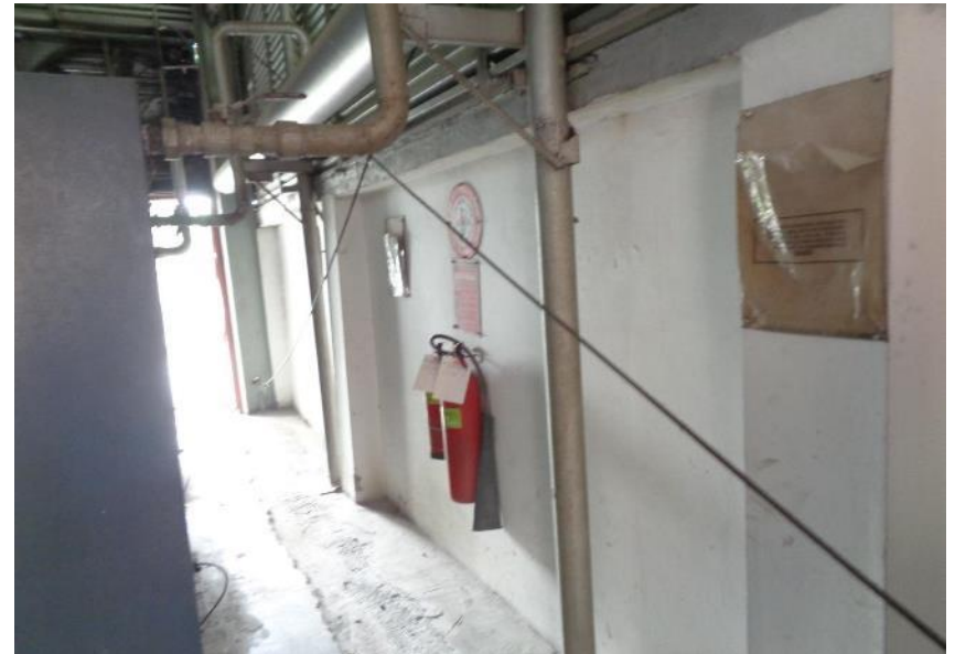
Loose cable bracing (Compressor Shed)
