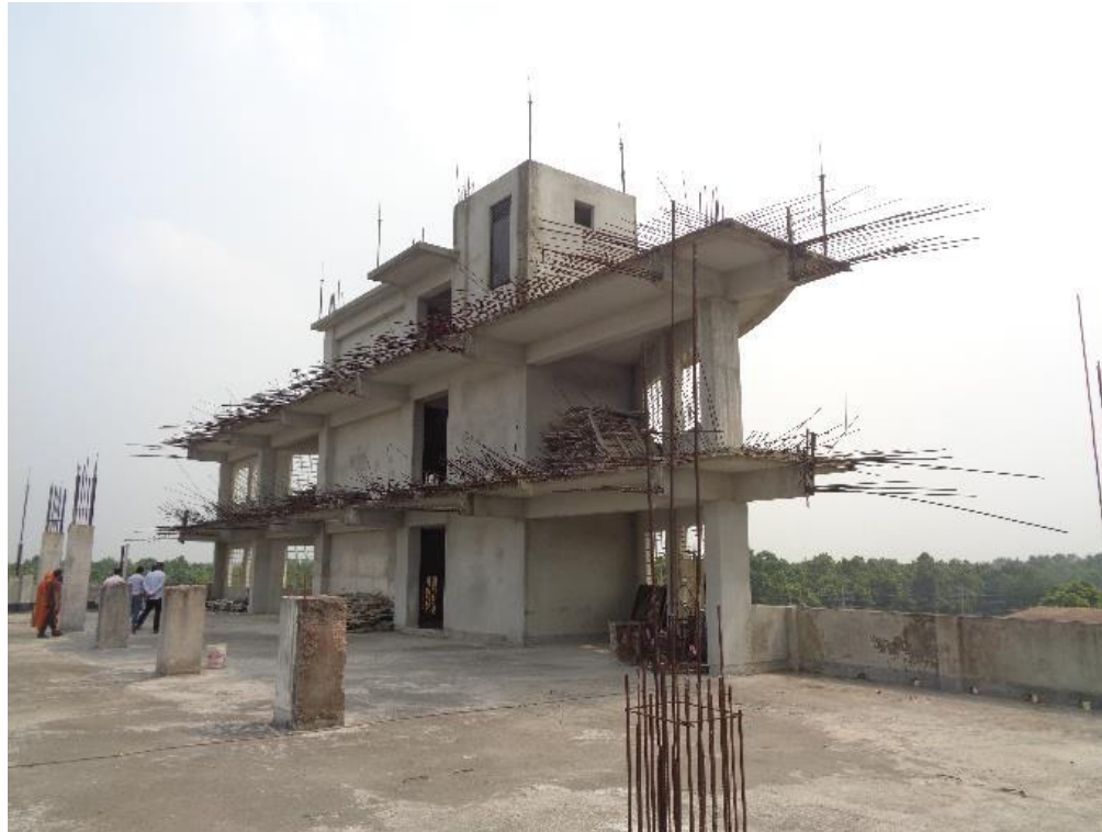
Exposed reinforcement left at roof (Main Building)
