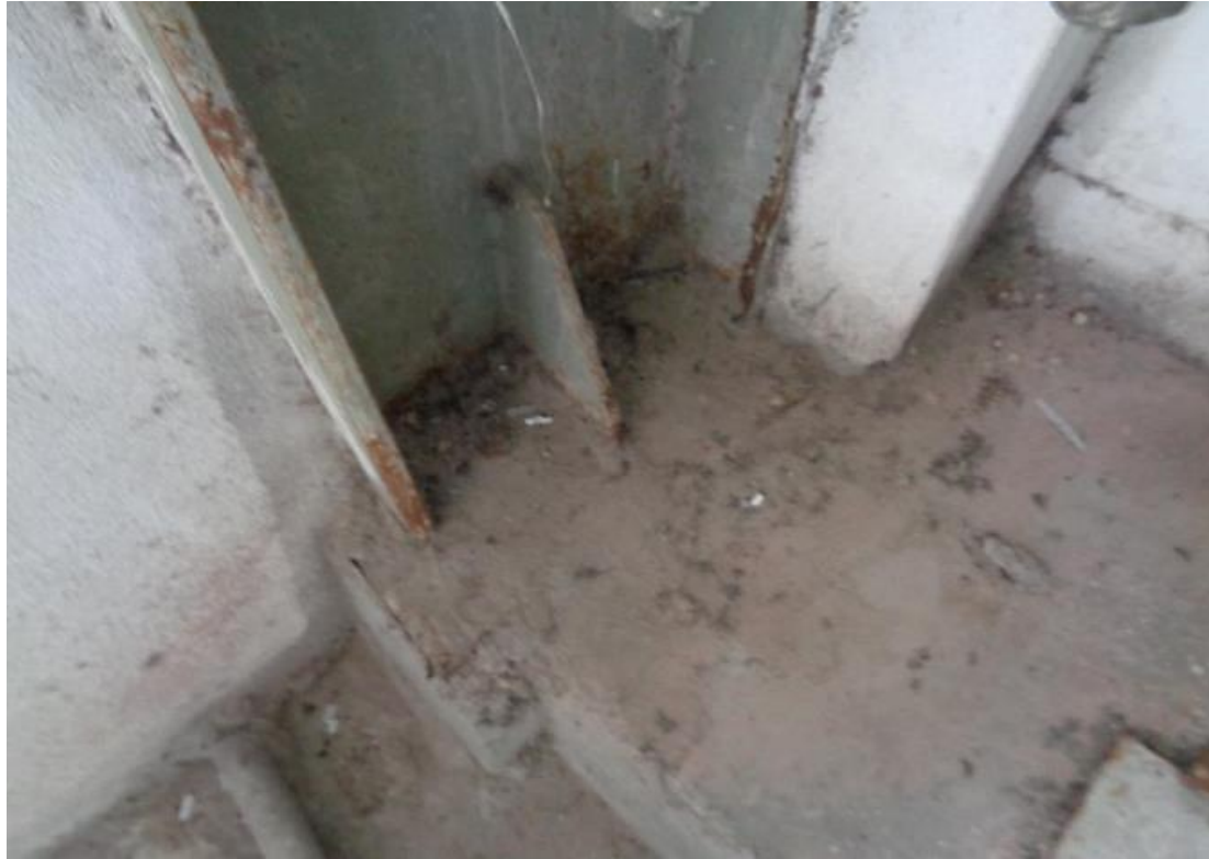
Corrosion on steel column (Compressor Shed)
