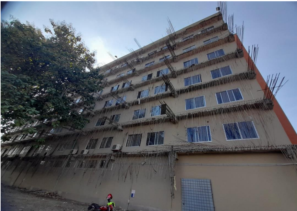
Projected reinforcement left at east side which indicates possible future horizontal expansion
