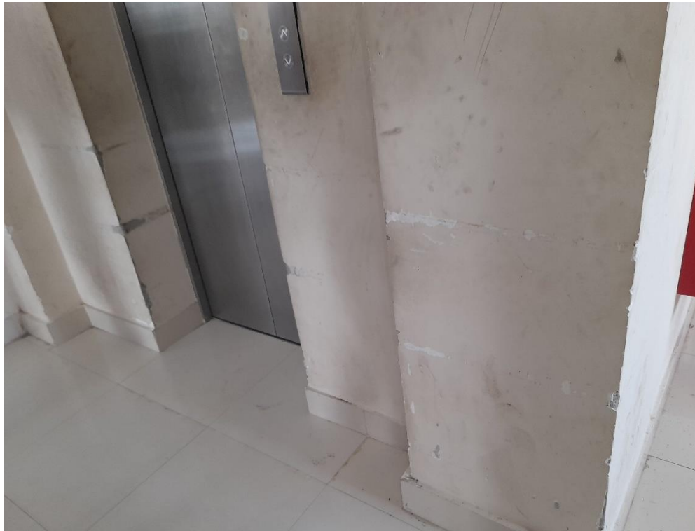
Affected columns at lift zone
