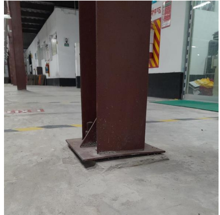
Gap between baseplate & pedestal joint
