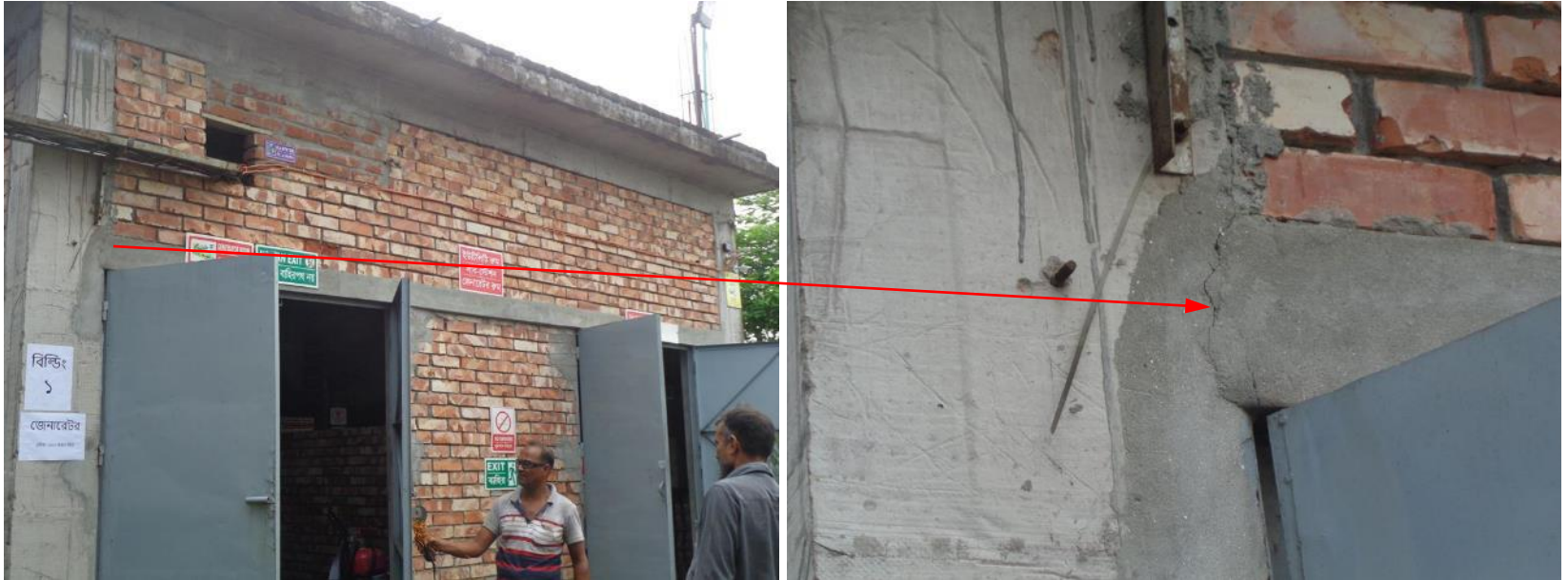
Hairline crack at the lintel-column joint over the door
