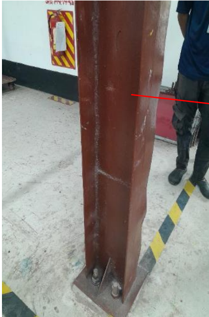
Distorted steel column
