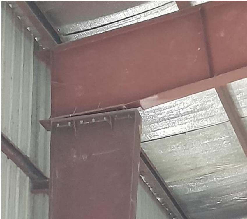
Gap between rafter and steel column joint
