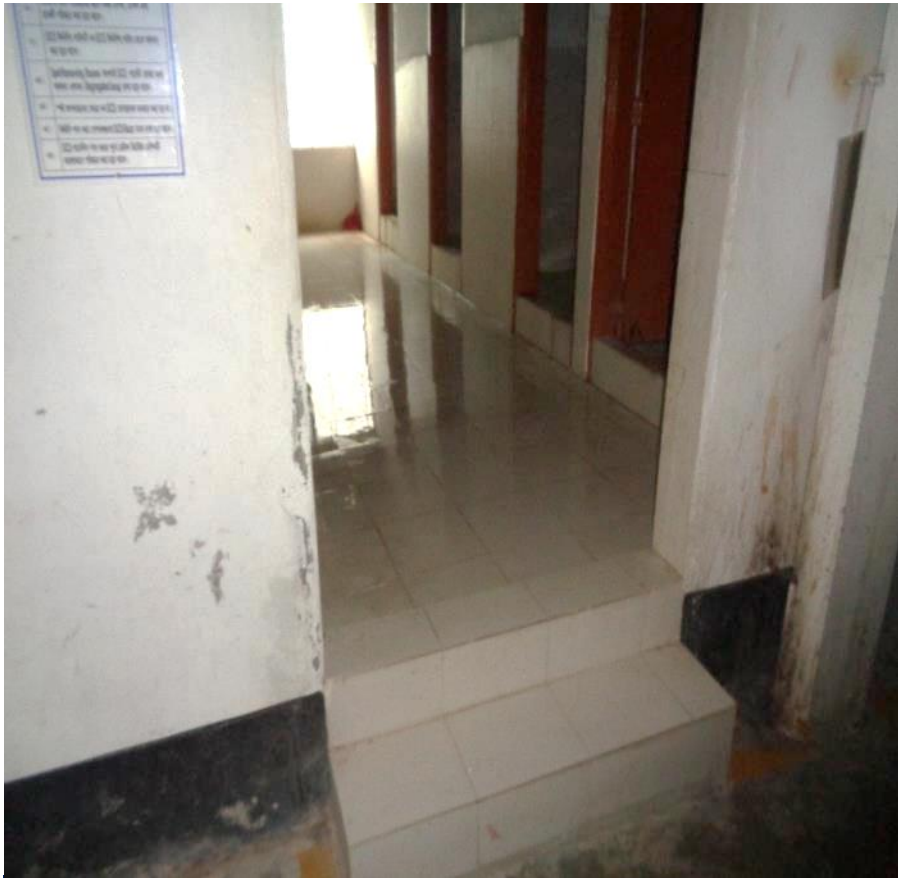
300 mm Build up found at toilet area
