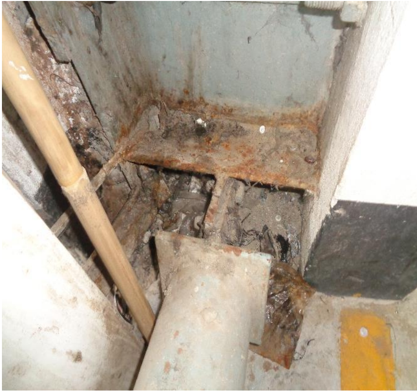
Corrosion on steel members
