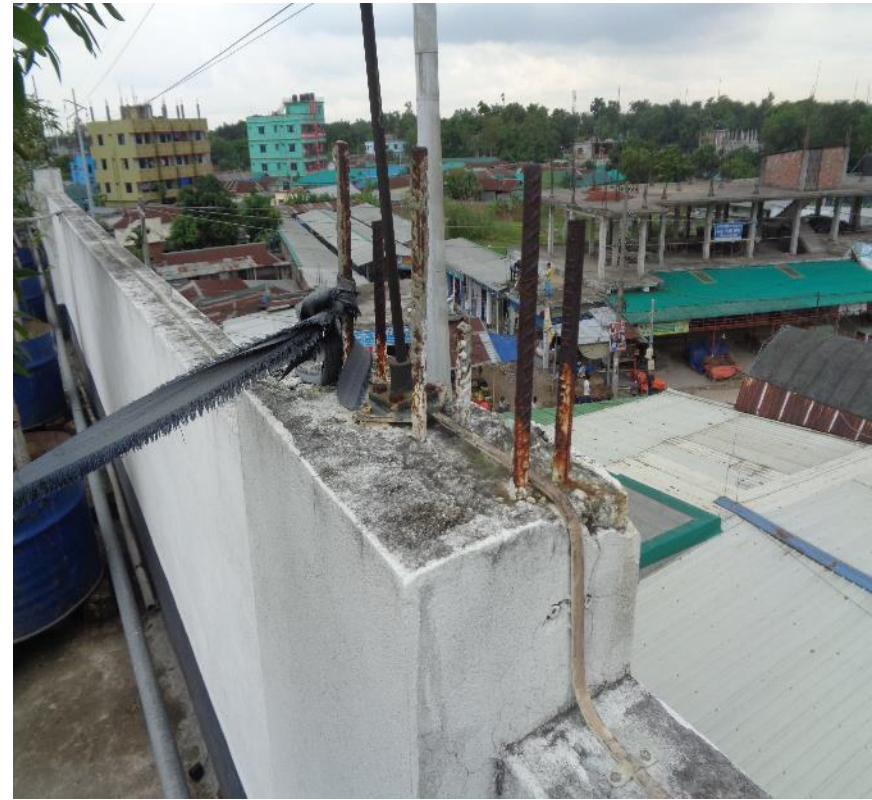
Corrosion on exposed rebar
