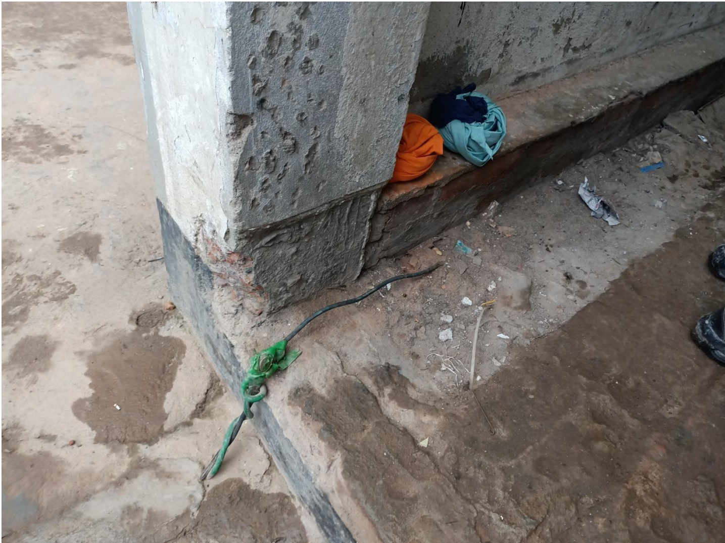
Bricks chips in column
