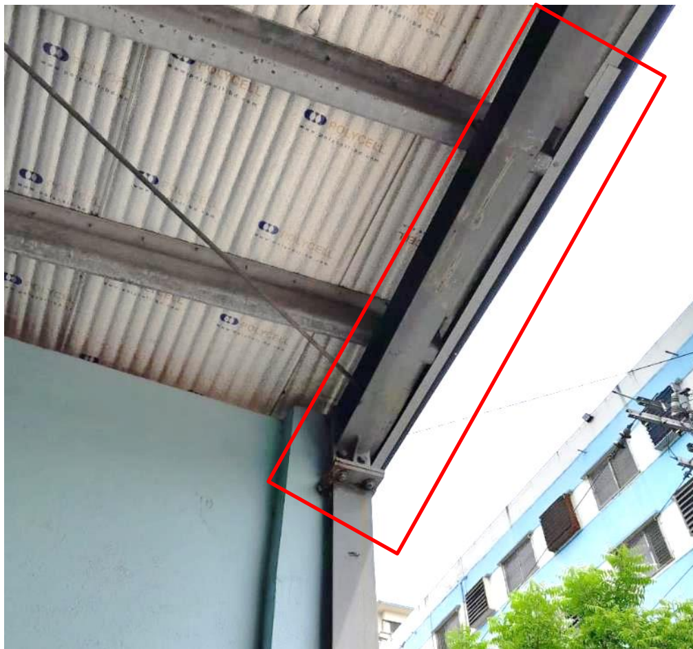
Corrosion in steel members
