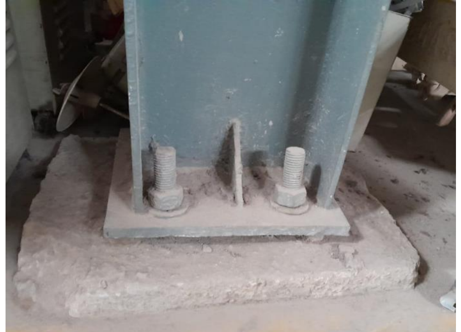
Connection gap in baseplate joint
