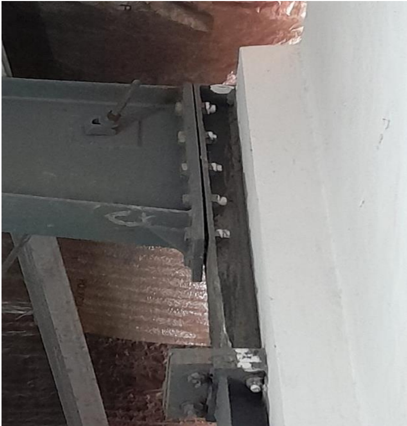
Connection gap in steel column-rafter joint
