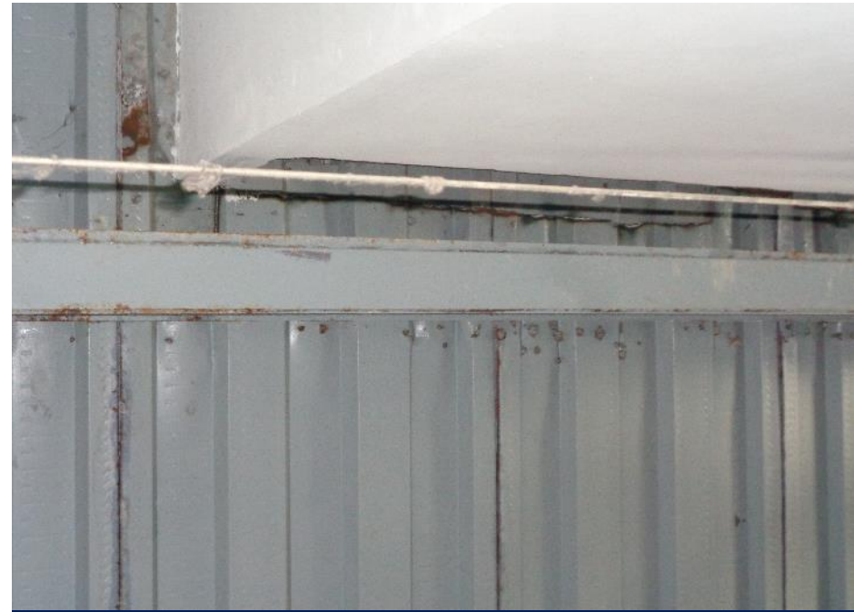
Highlighted beam was not found on site
