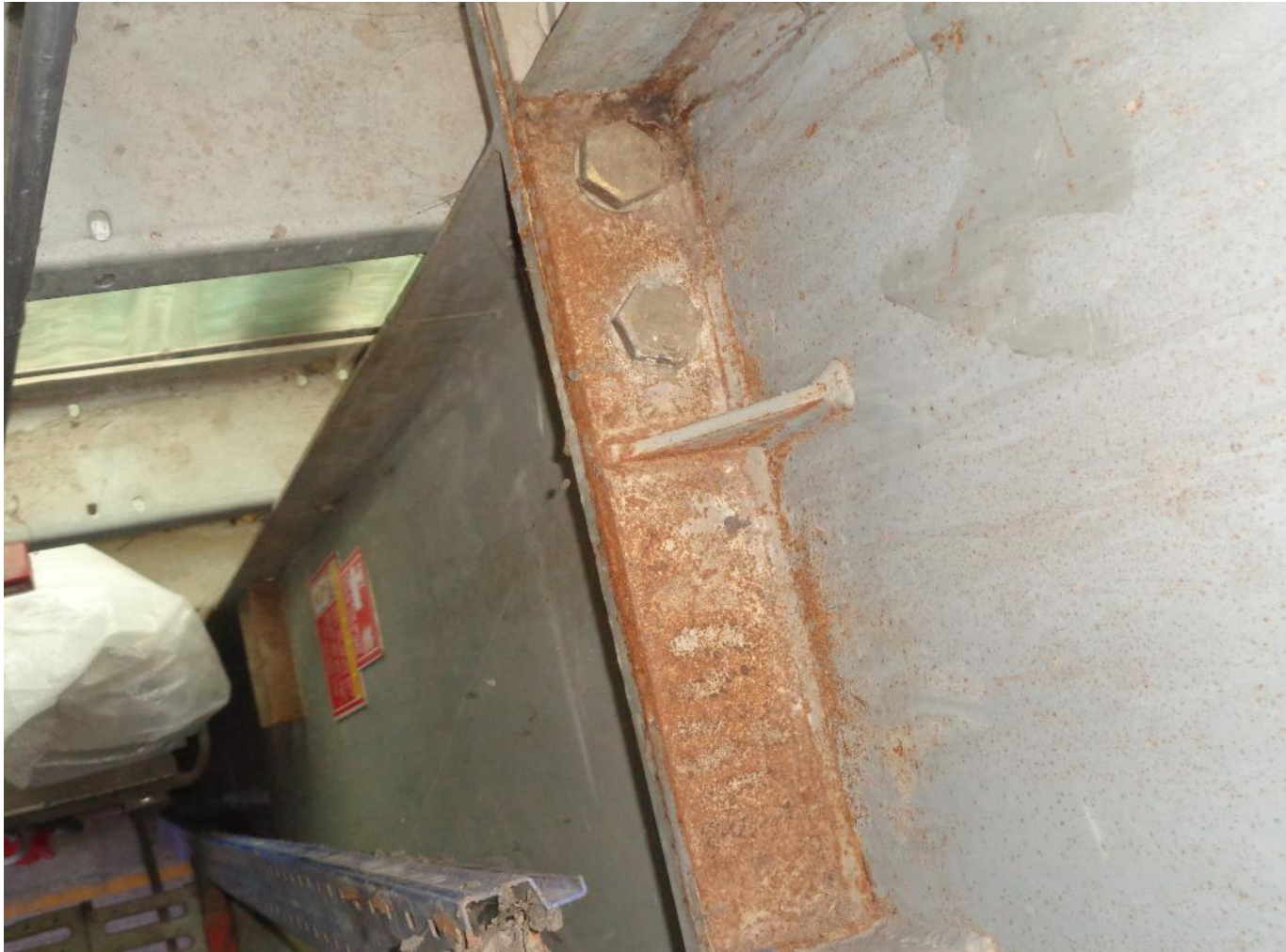
Corrosion on steel column
