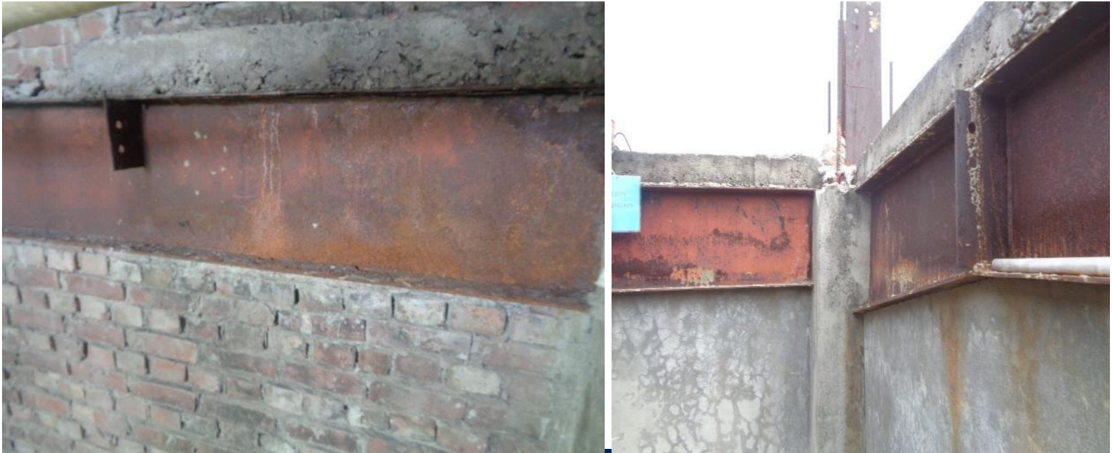
Corrosion on steel beam at staircase
