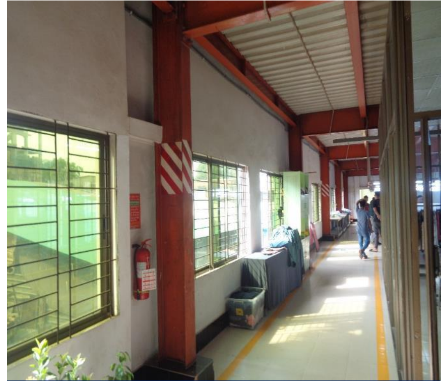
No bracing or any lateral load resisting system along N-S direction
