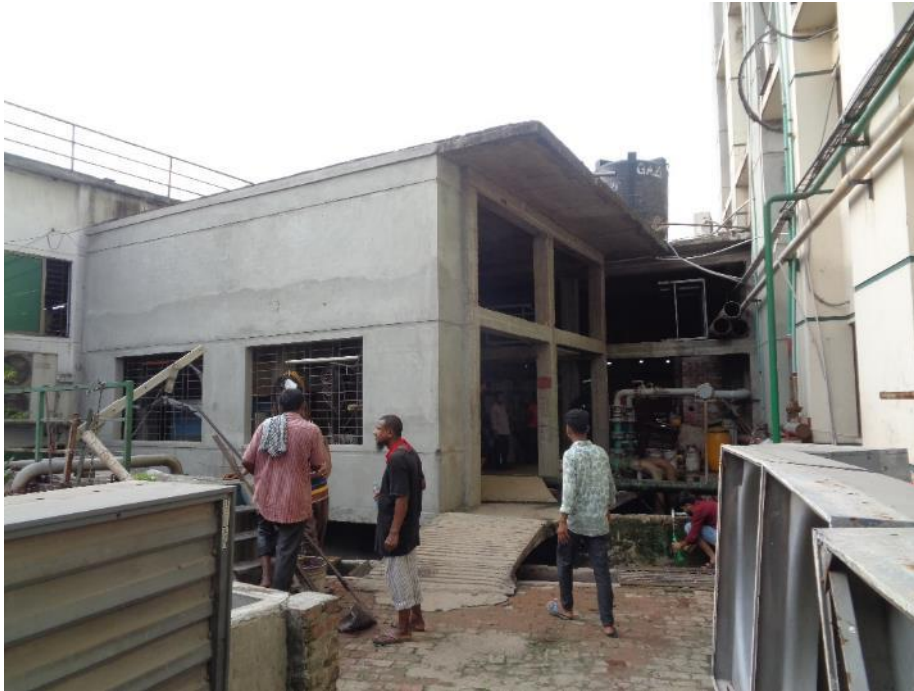
Fire Pump House
