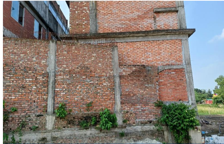
Vegetation grown on the facade wall
