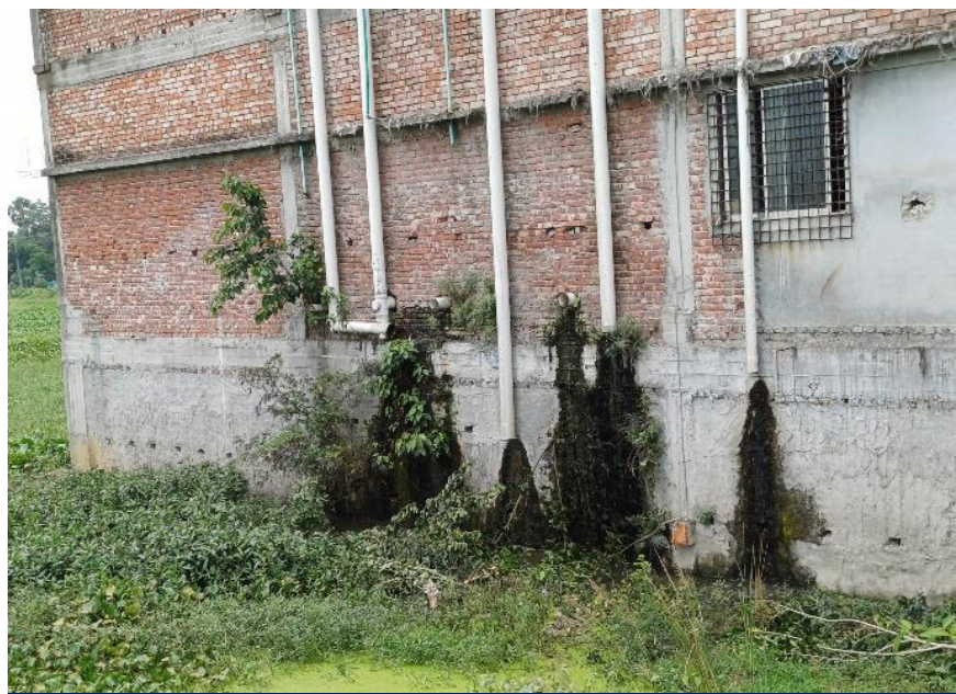
Vegetation on facade wall damp grade-beam due to exit of down pipe
