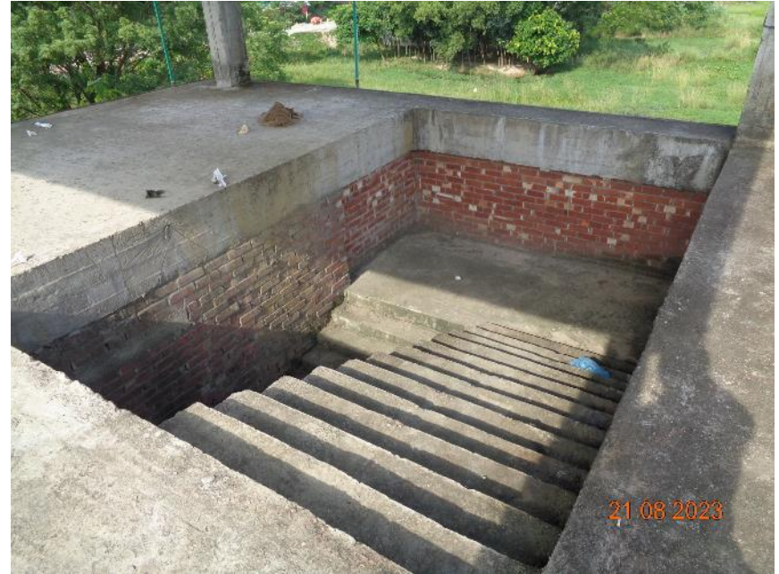
Falling hazard at stair
