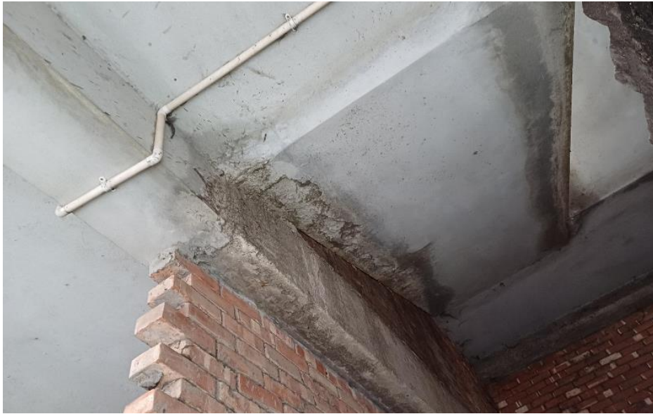
Dampness in stair area
