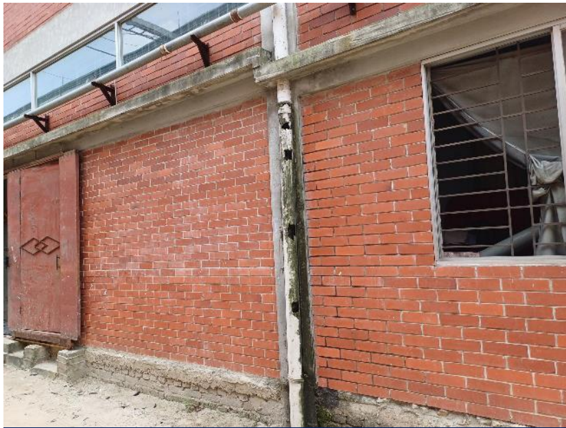
Dampness in column and grade beam due to broken PVC pipe
