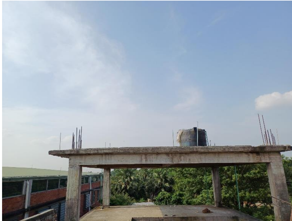
Undocumented water tank at roof of stair
