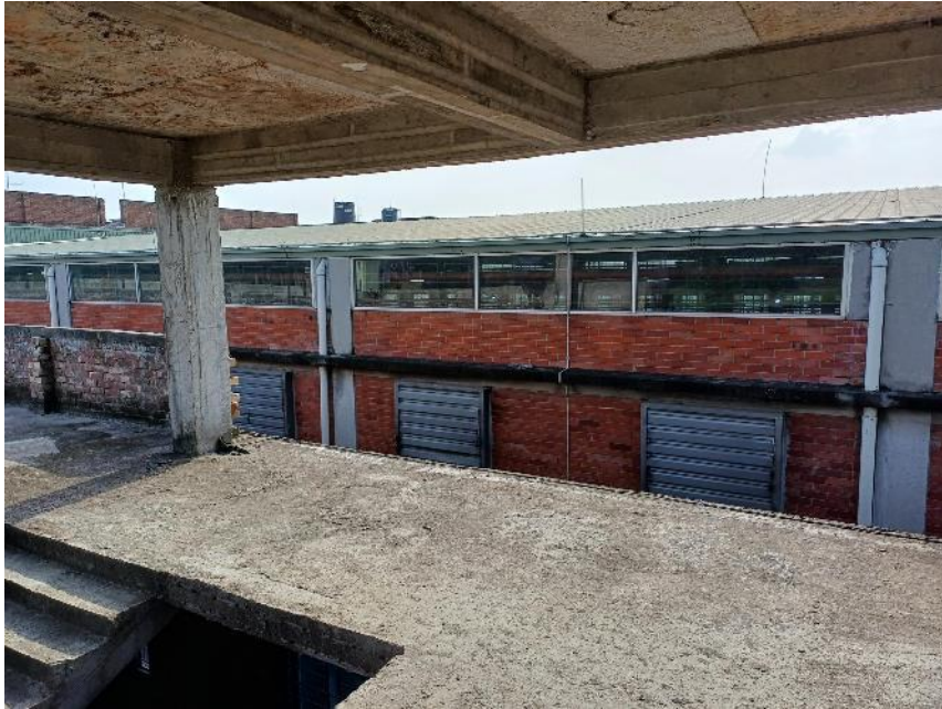
Falling hazard at roof
