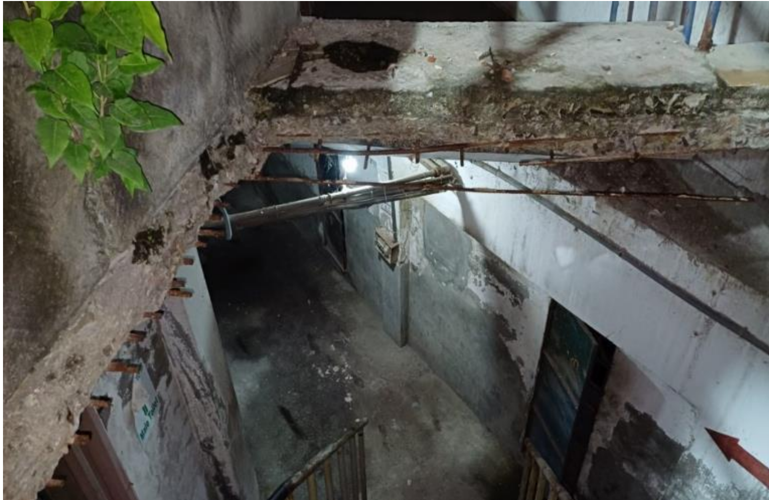
Exposed reinforcement left at mezzanine level
