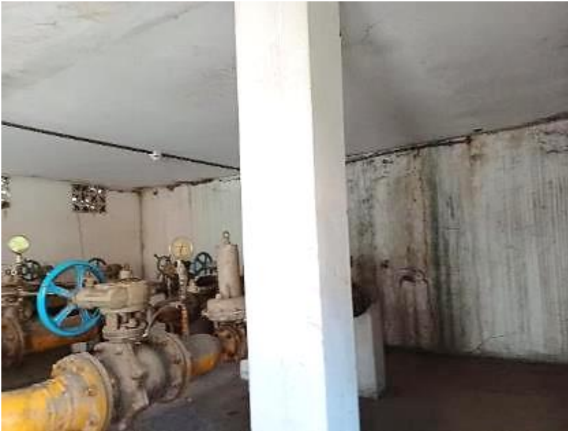
Dampness on wall and roof slab
