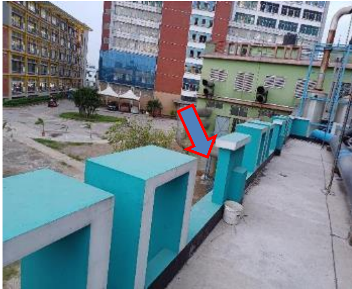
Discontinuous parapet on roof
