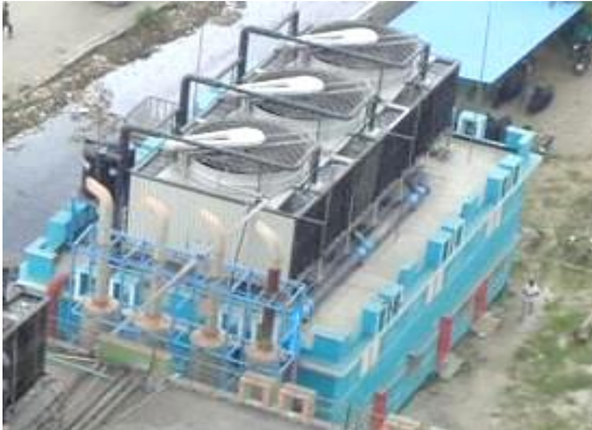
Heavy loading on roof
