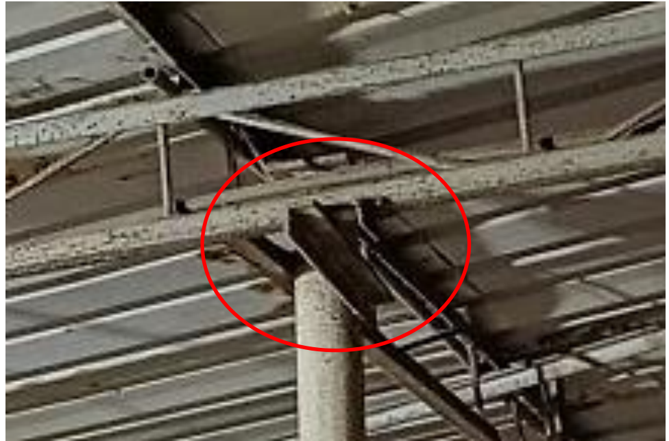
Poor connection of truss to steel pipe
