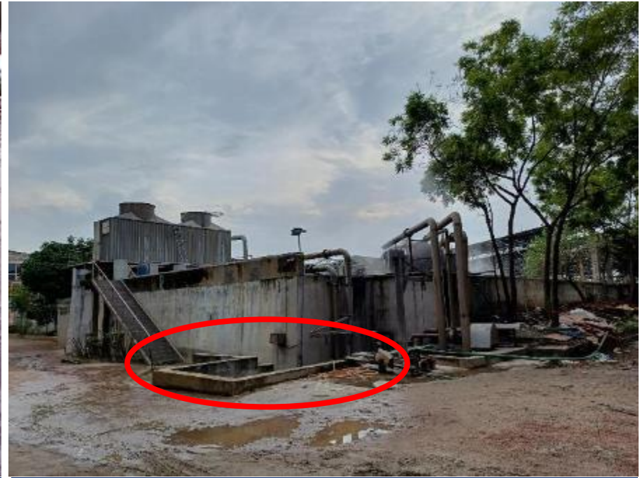
Lack of railing and falling hazard screening area
