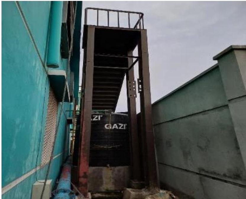
No vertical bracing provide for the stair
