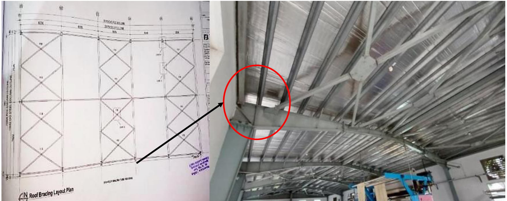
Bracings connected apart from column-rafter joint
