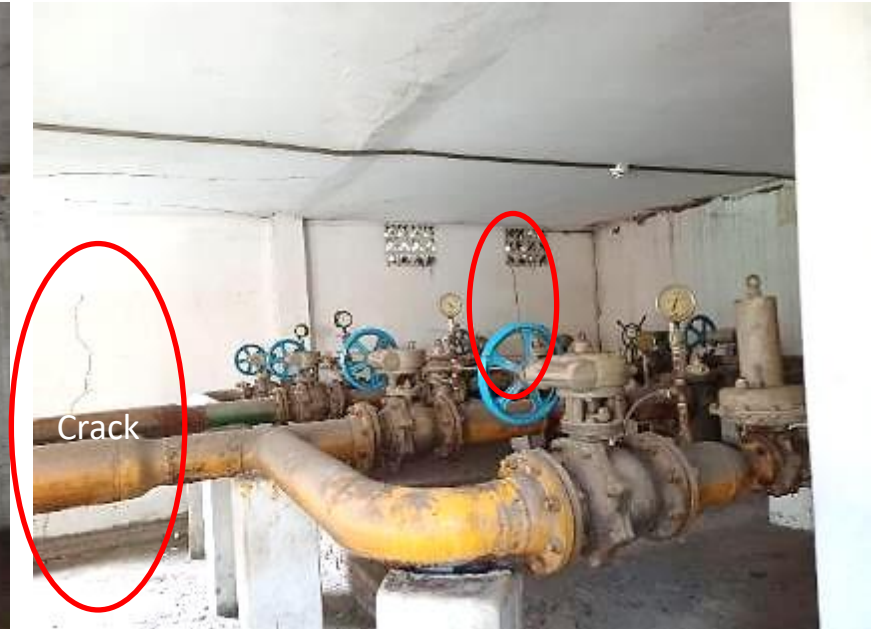
Crack on brick wall
