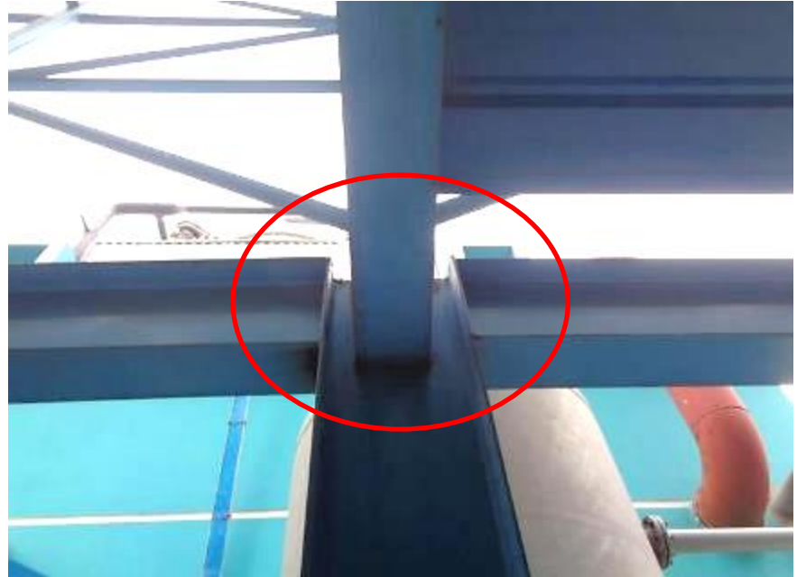
Discontinuity of top plate in beam-column joint
