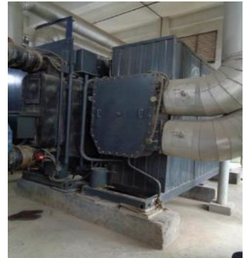
Source of loading: Chiller
