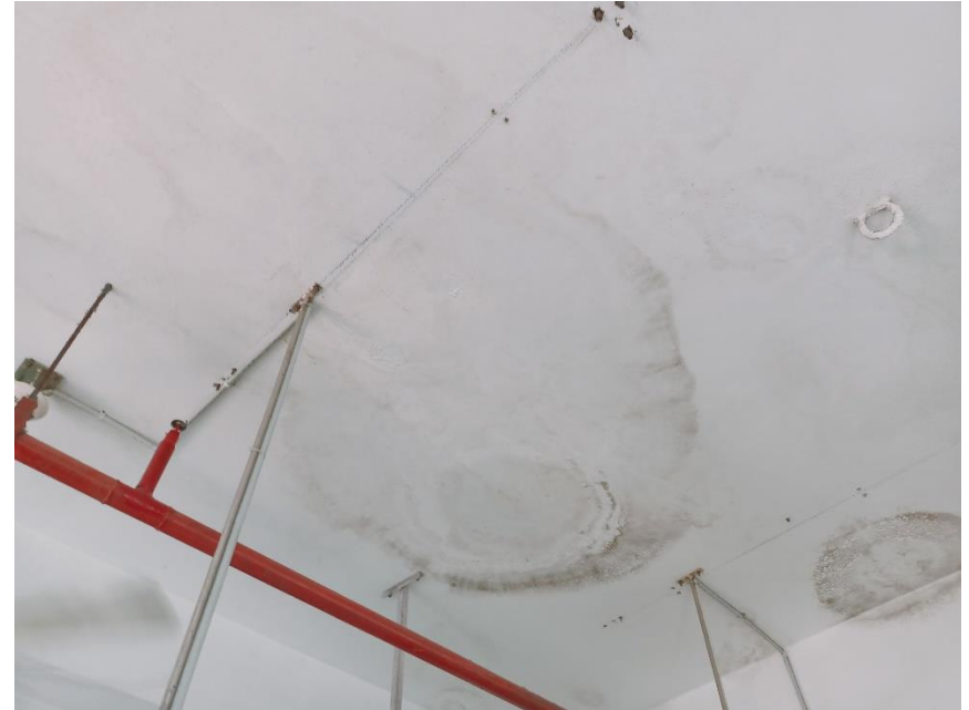
Dampness on slab soffit
