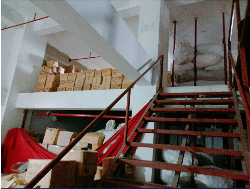
Racking platform on ground floor
