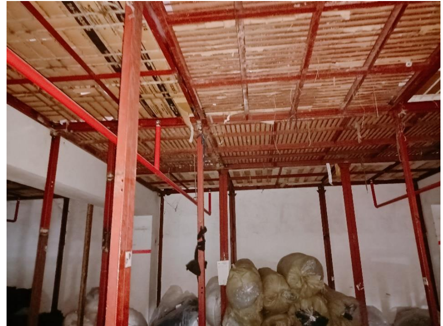
Apparently inadequate member & connection
