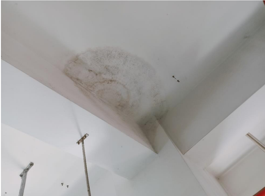
Dampness on slab soffit
