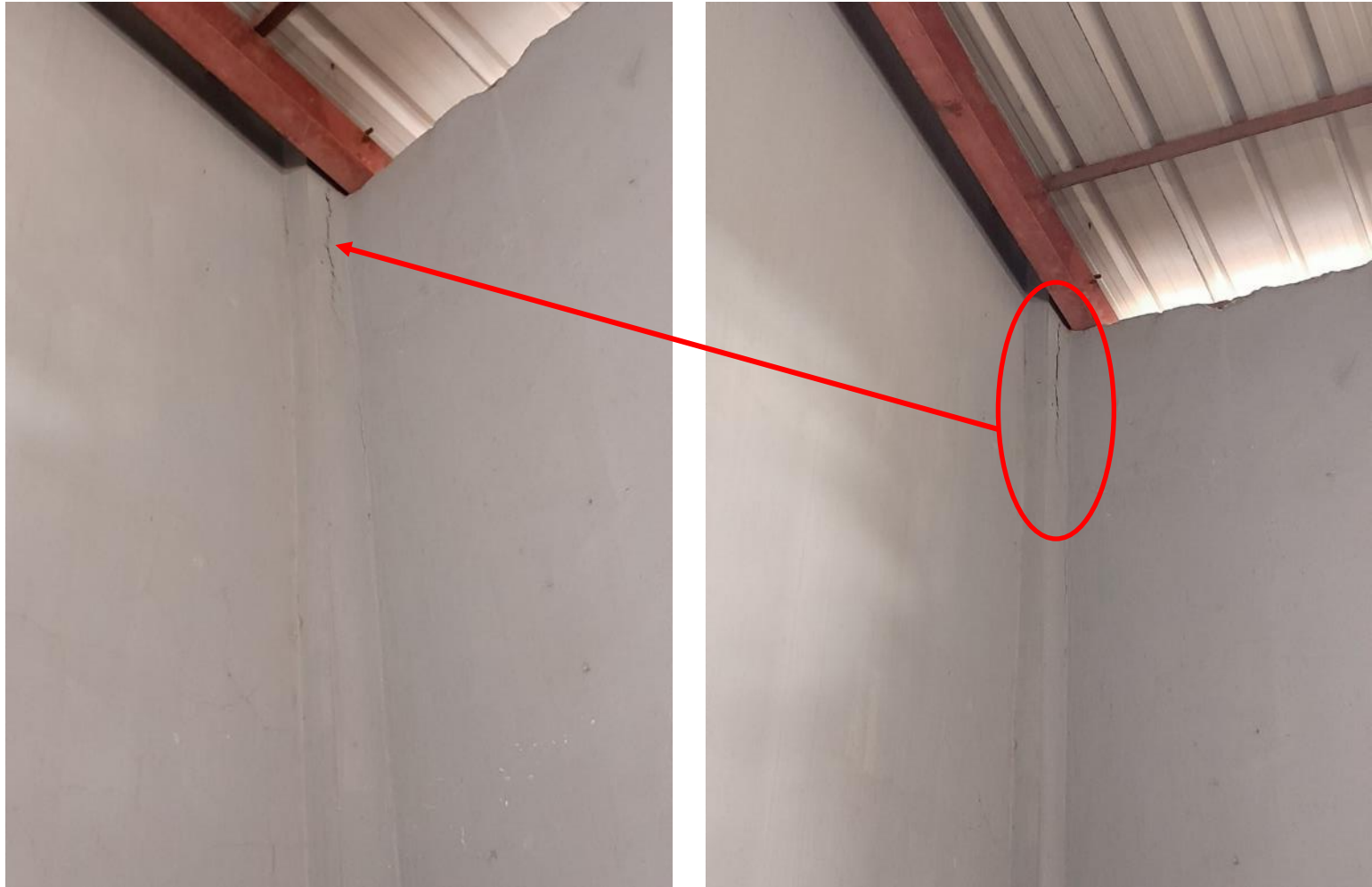
Crack on column surface at column-wall joint
