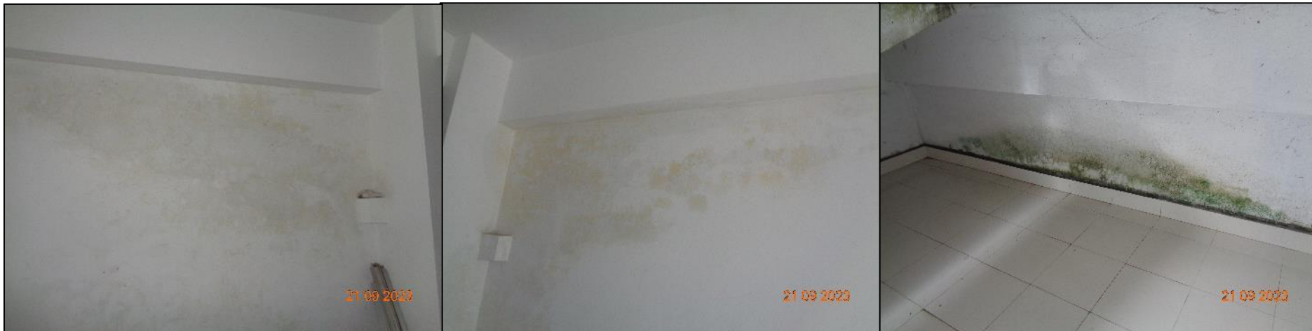
Dampness on Wall
