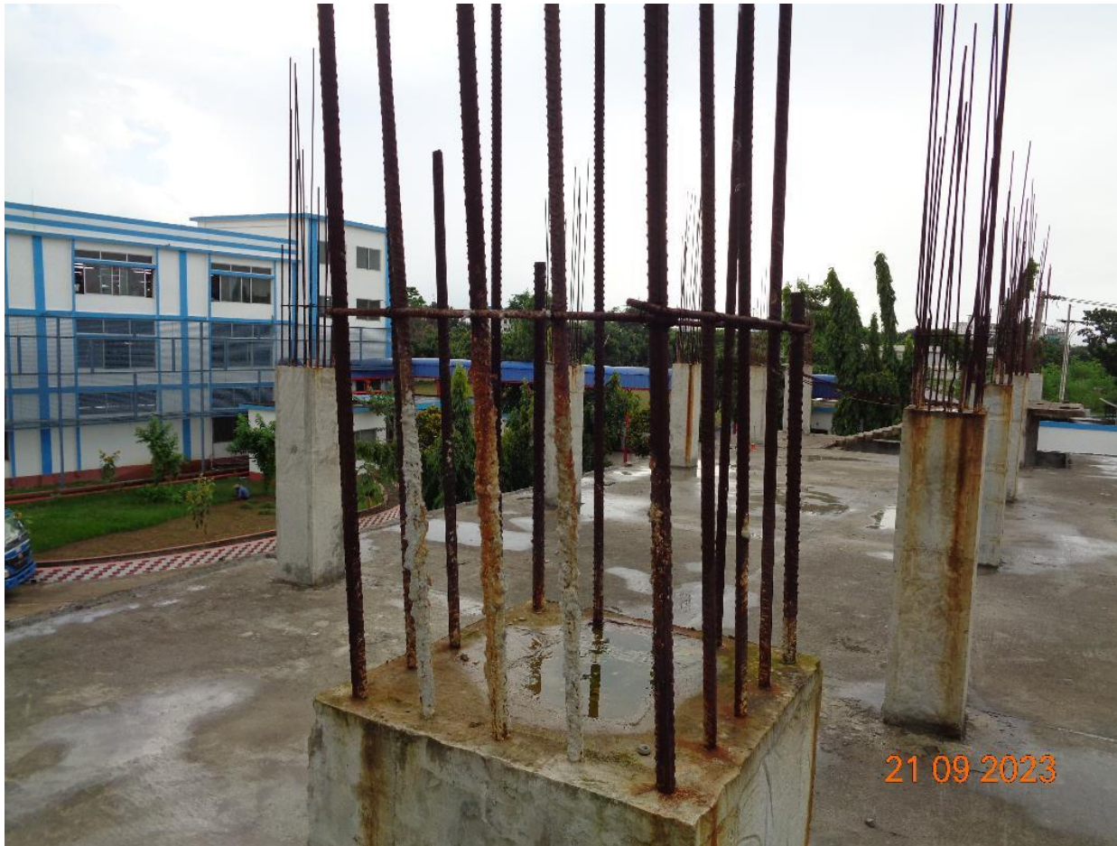
Exposed rebar of Column
