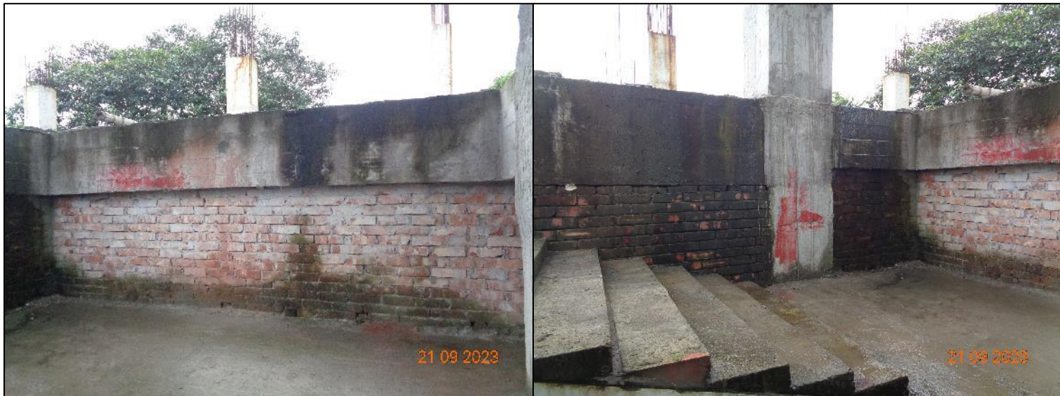
Dampness on beam
