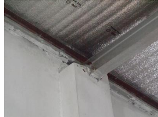
Apparently inadequate member & connection
