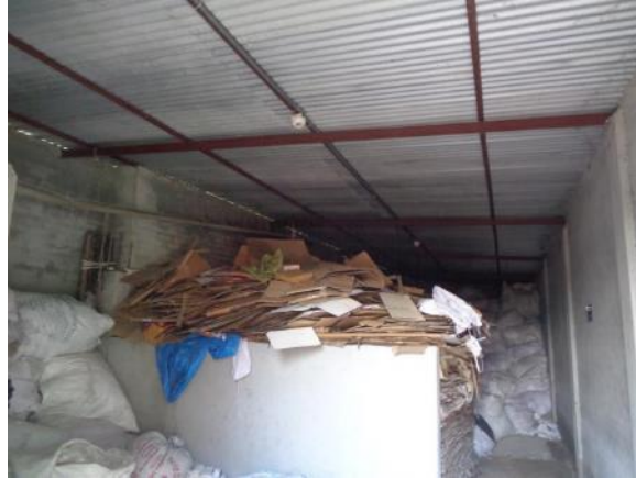
Apparently inadequate rafter
