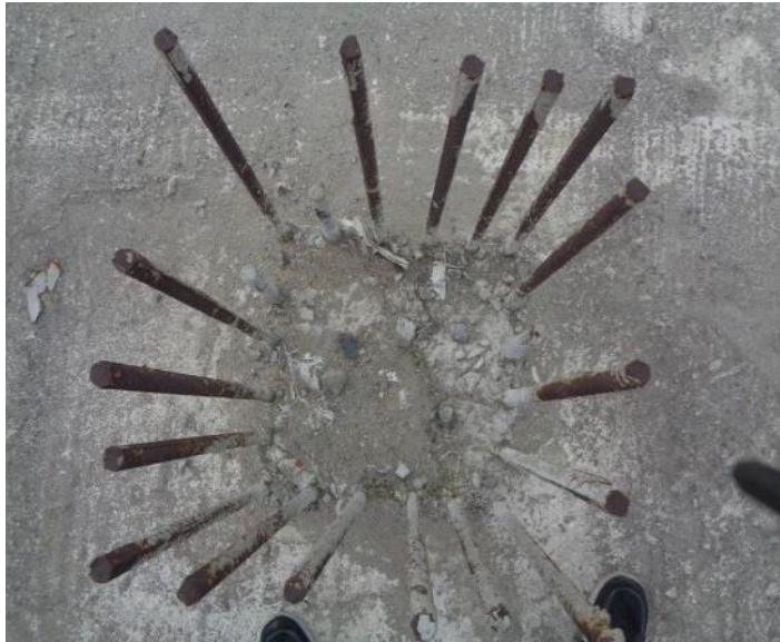
Exposed rebar on roof
