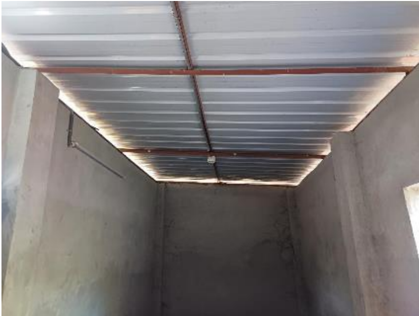
Inside of STP shed
