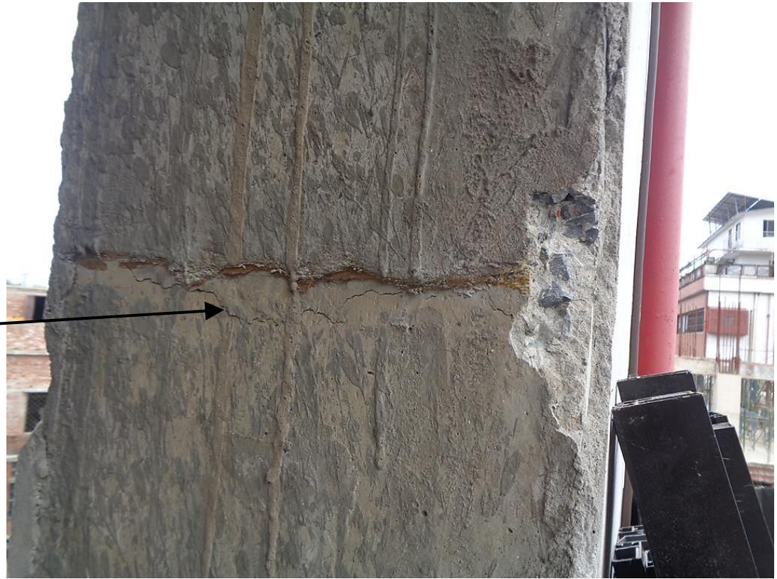
Crack in stair column at roof level
