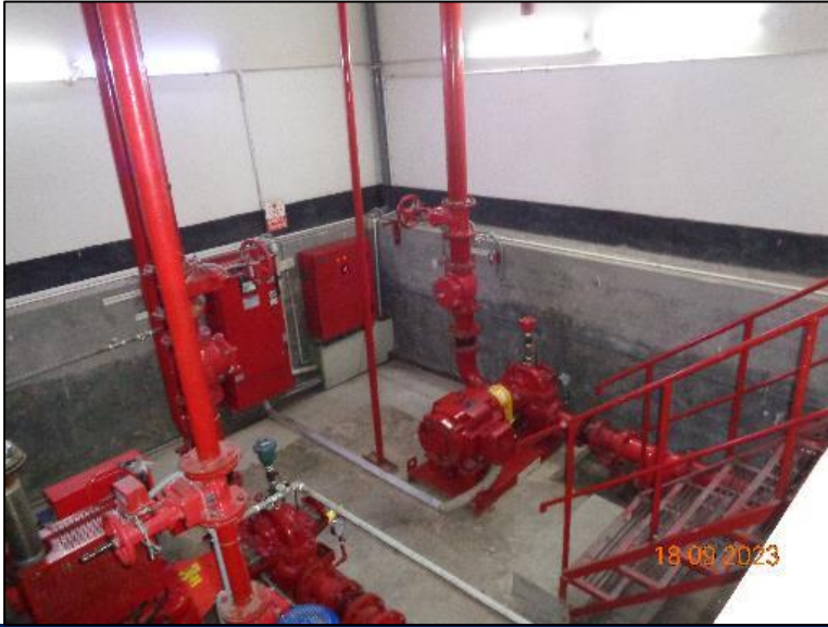
Fire pump room below ground level
