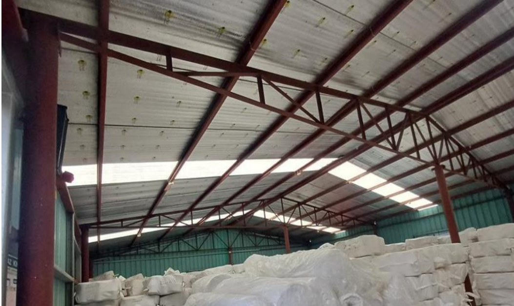
No load transfer media & bracings at roof
