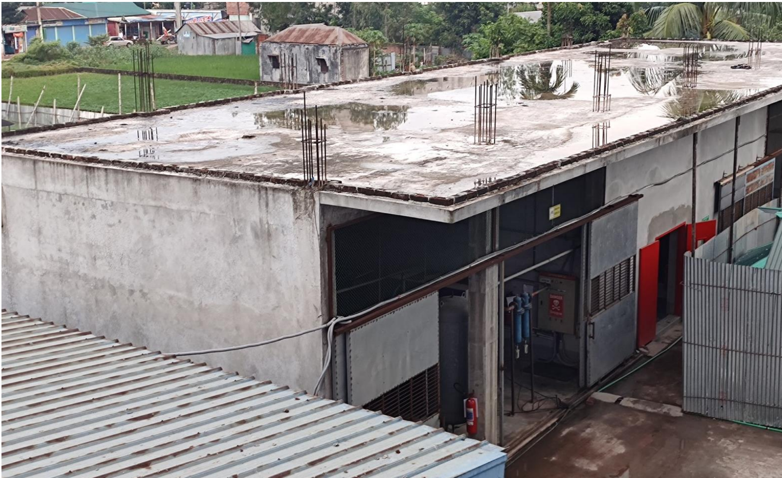
Water ponding and exposed rebar on the roof.
