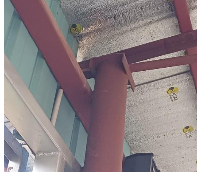
Improper connection between steel column and steel roof
