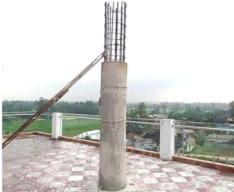
Exposed rebar at roof top column
