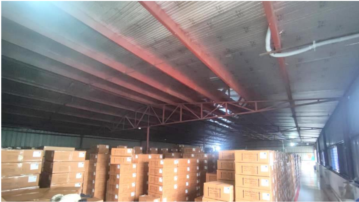
Absence of load transfer media along transverse direction and absence of bracing
