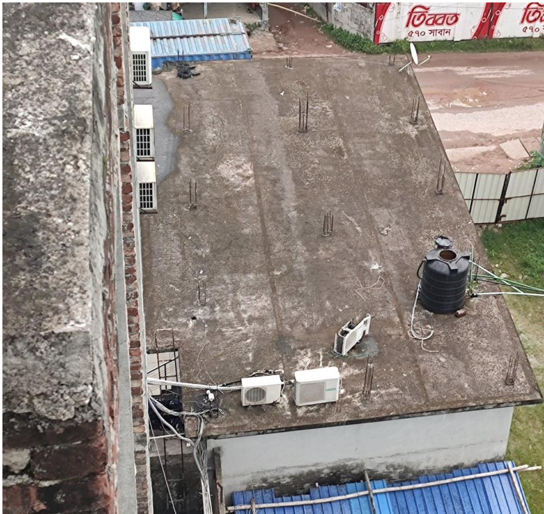
Exposed rebar on roof
