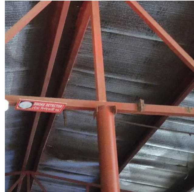
Improper connection between steel column and steel roof
