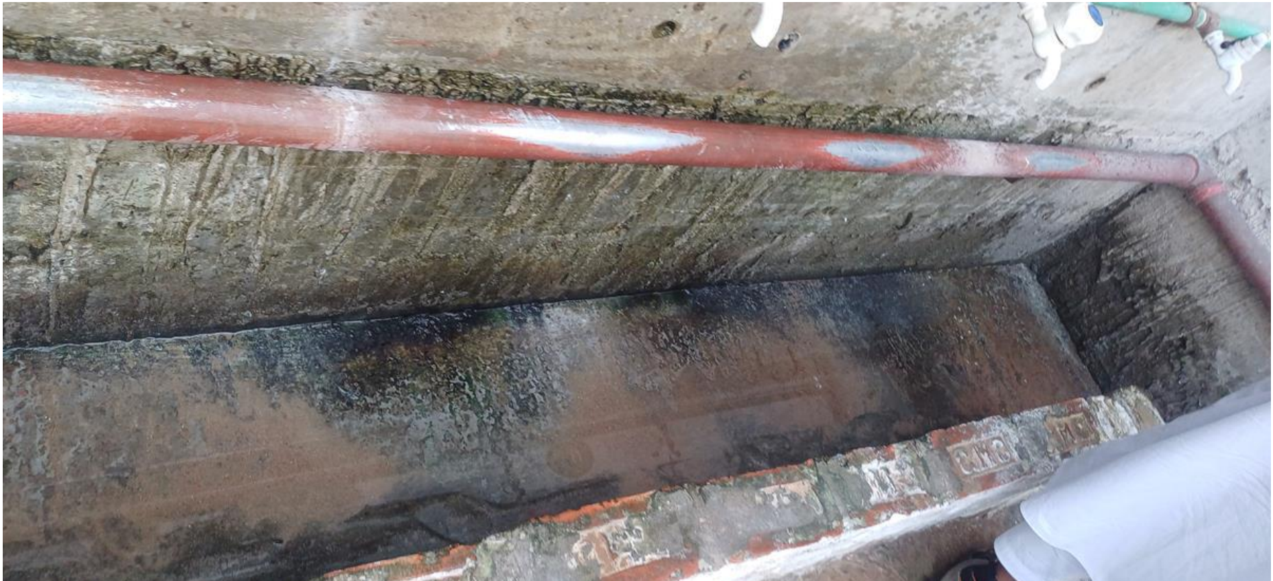
Dampness on outer face of shear walls
