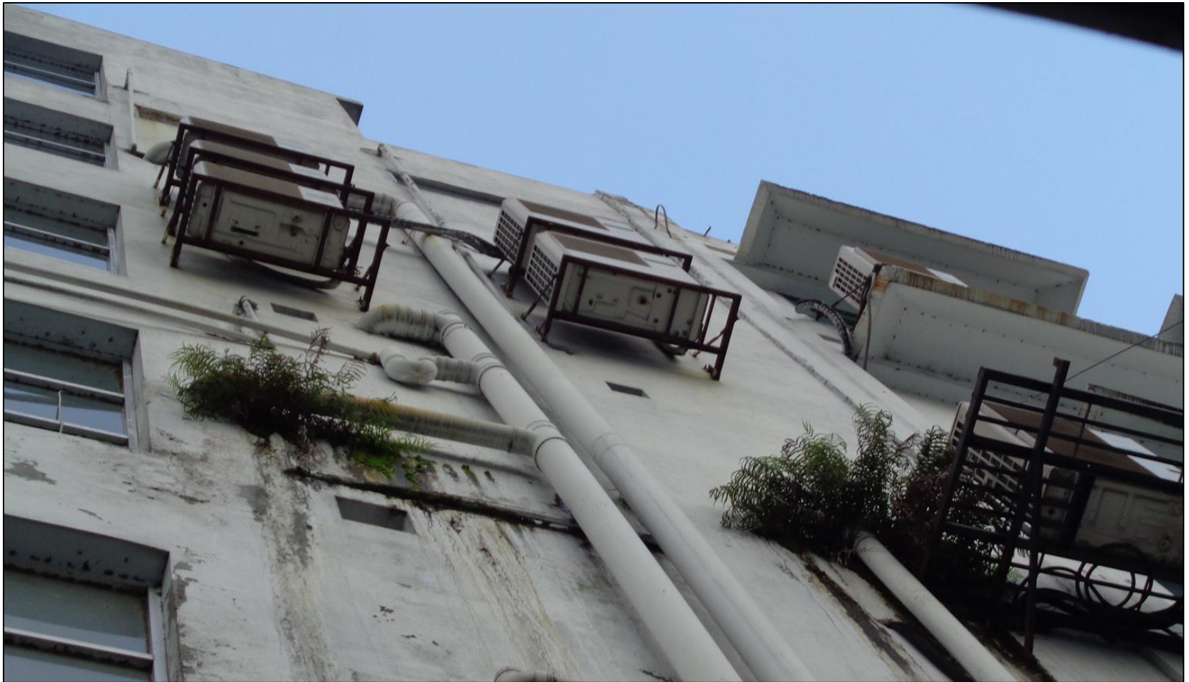
Dampness and vegetation on building façade.
