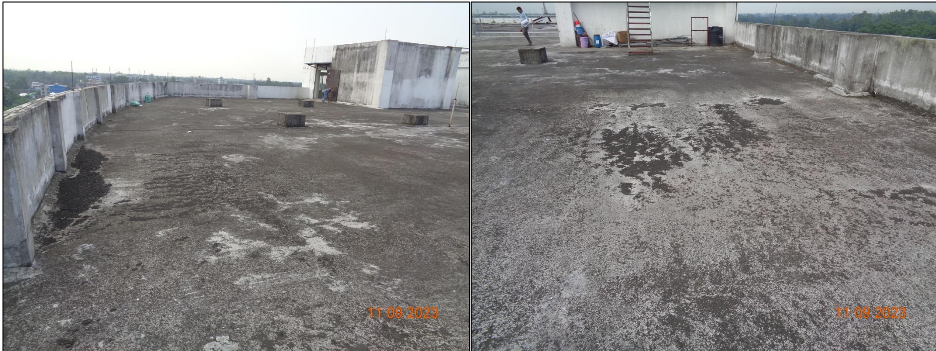
Signage of water ponding on roof slab
