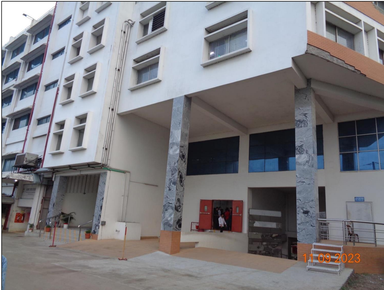
Columns having no barrier/protection at ground floor
