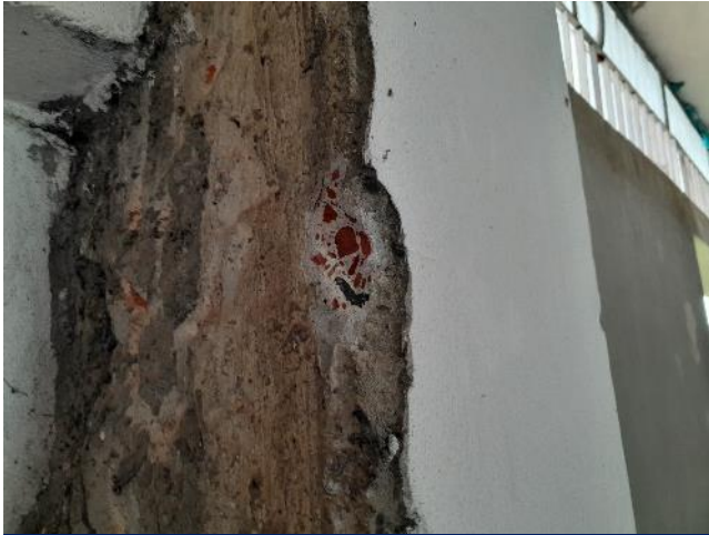
Brick aggregate in column of Utility Building
