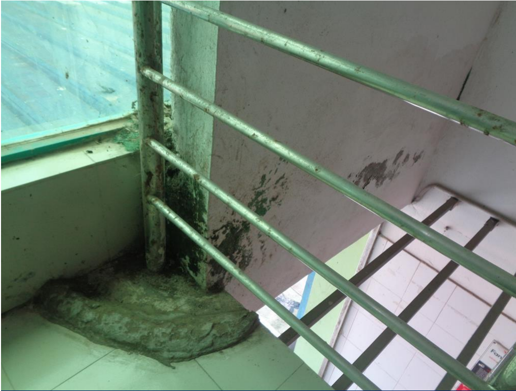
Dampness at peripheral brick wall
