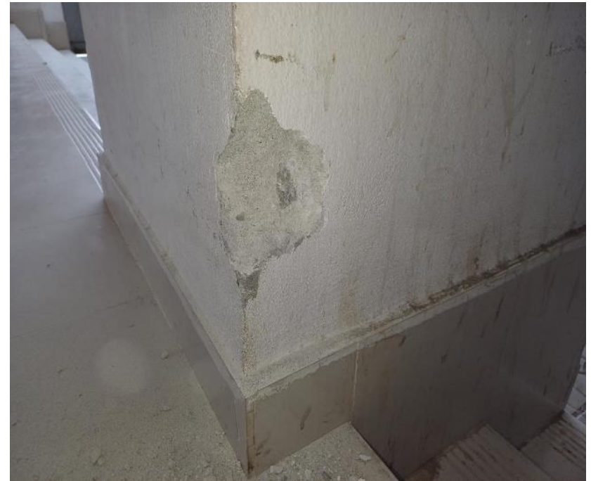
Stone chips in column
