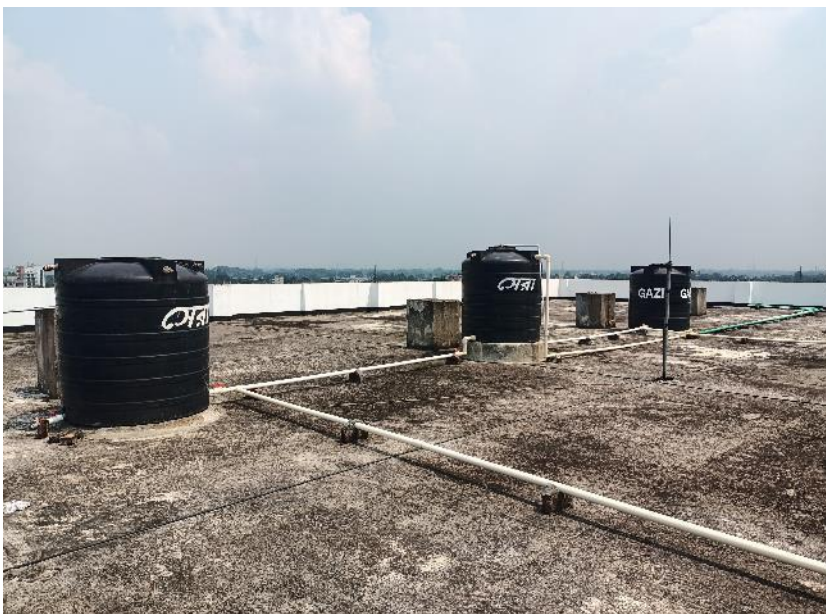
Plastic water tank not braced
