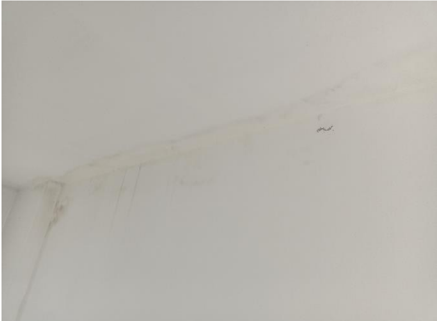
Dampness on slab soffit
