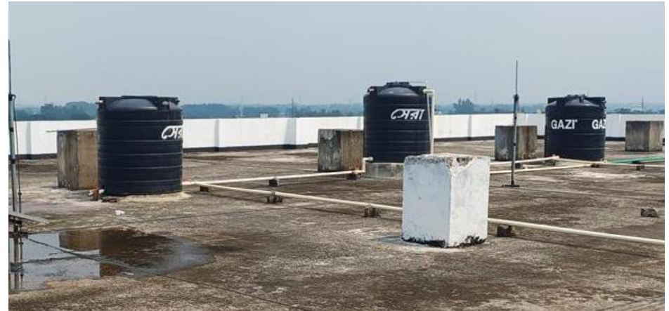
Undocumented water tank
