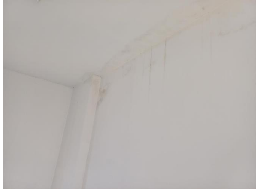
Dampness on slab soffit
