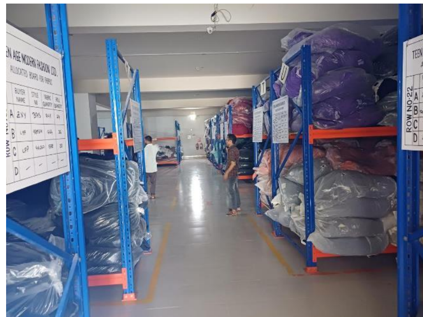
Non-anchored storage rack at several floors
