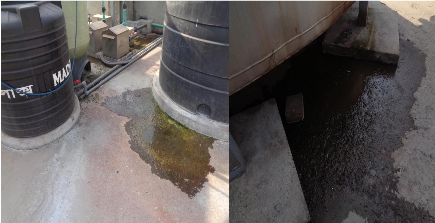
Dampness on roof slab
