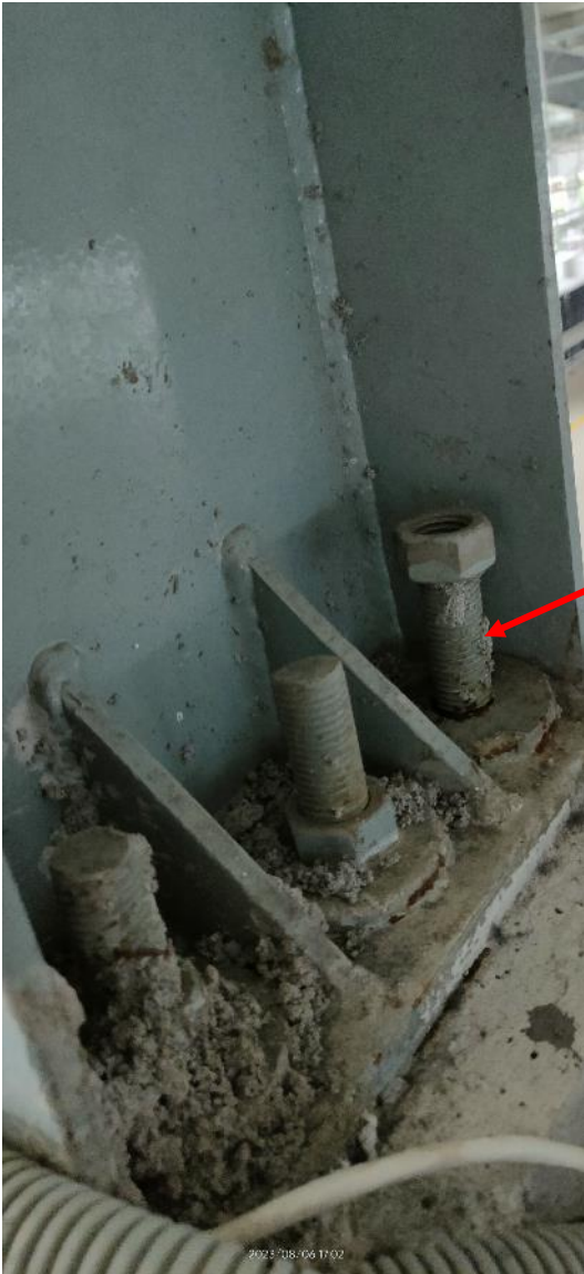
Loose bolt in baseplate
