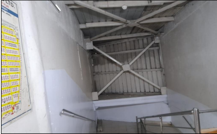
Bracing on 3 rd floor not shown in the retrofitting drawing
