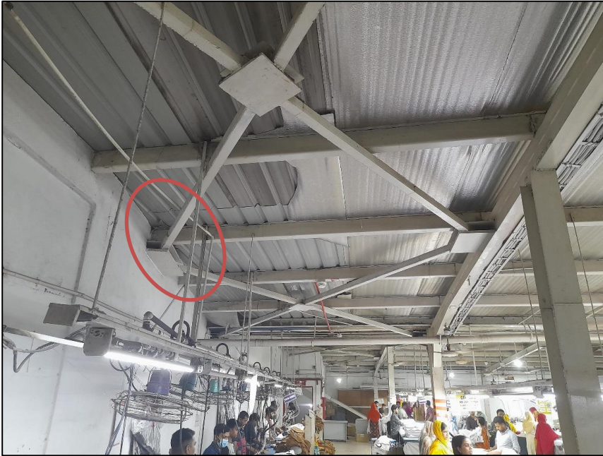
Connection plates inserted into adjacent RC building instead of steel edge rafter
