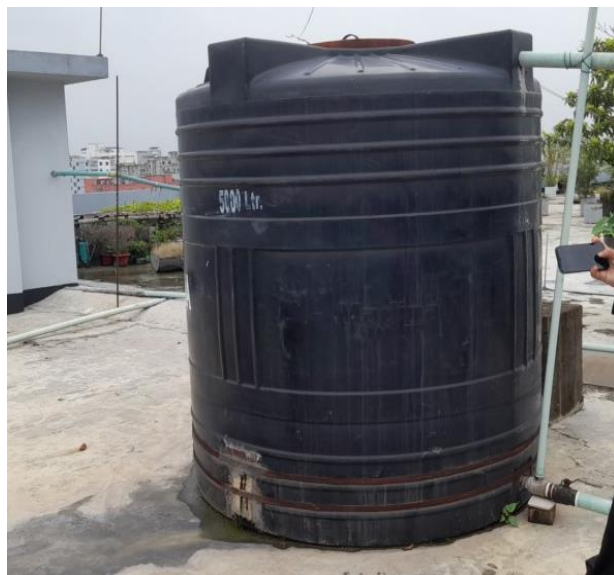
5000L water tanks on Roof
