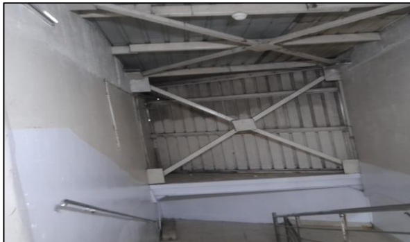
Bracing on 3 rd floor not shown in the retrofitting drawing
