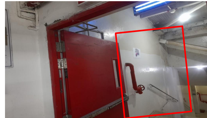
Vertical bracing at Grid-1-E~F near to 3 rd floor stair could not identified.
