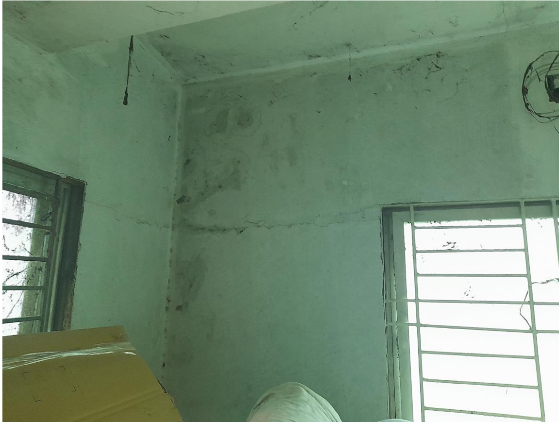
Dampness & crack on peripheral brick wall
