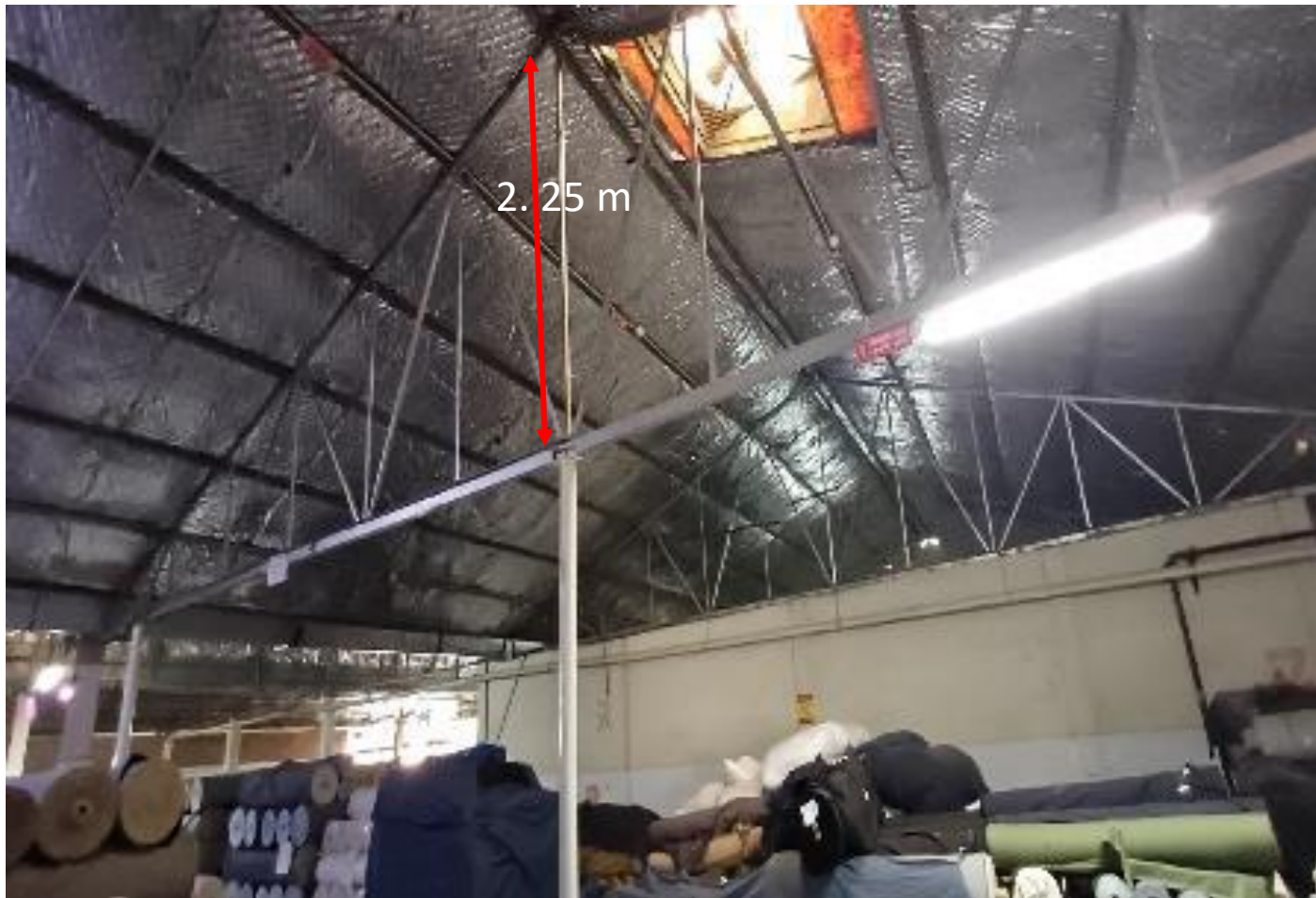
Absence of load transfer media (strut) and load resisting (bracing) system
