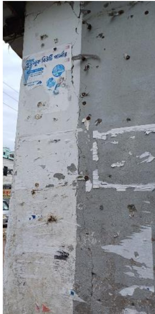
Crack on brick wall
