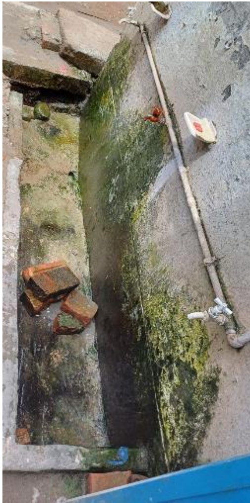
Dampness on wall at west
