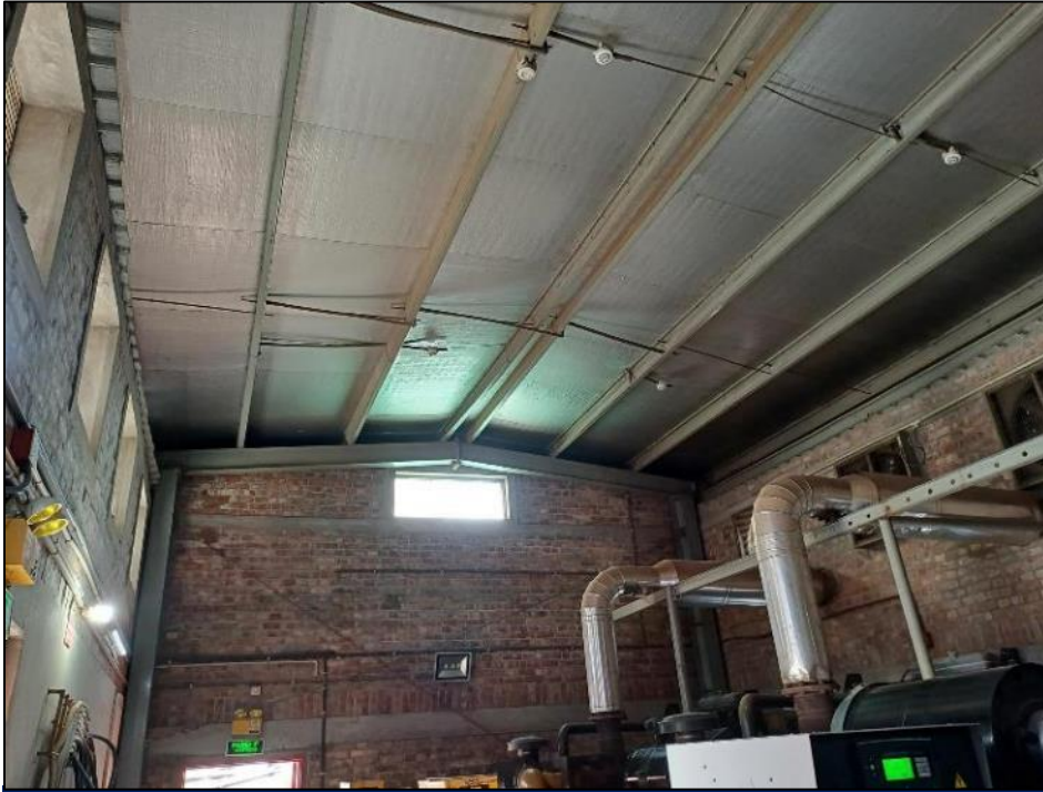
No load transfer media/roof bracing is provided
