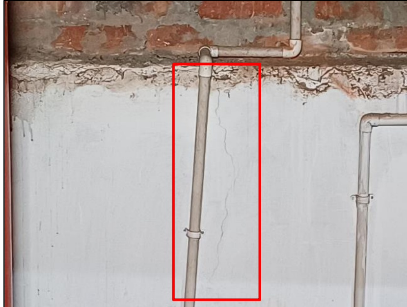
Retaining Wall Crack
