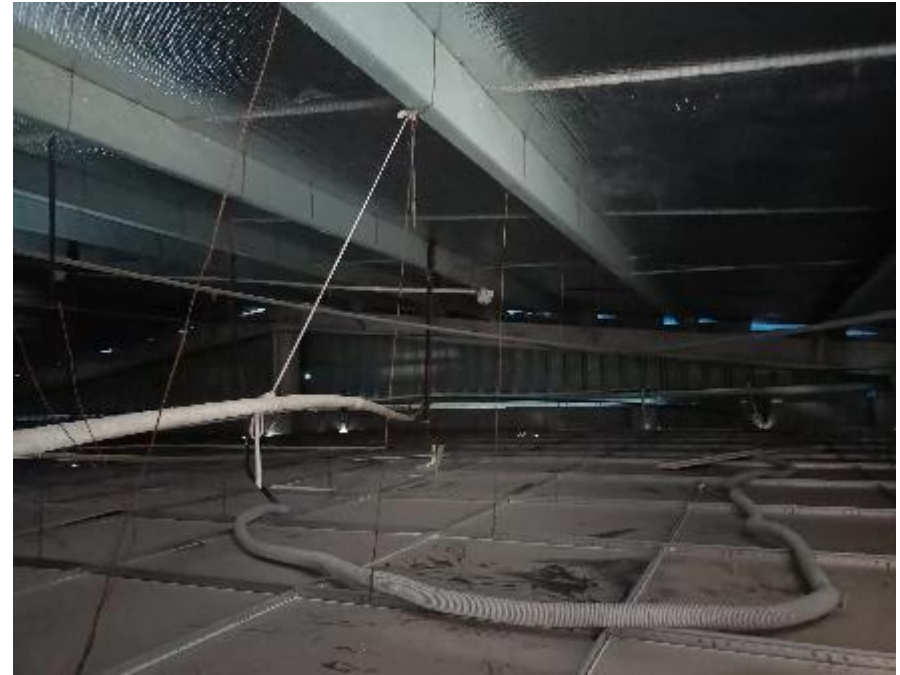
Loose cable bracing
