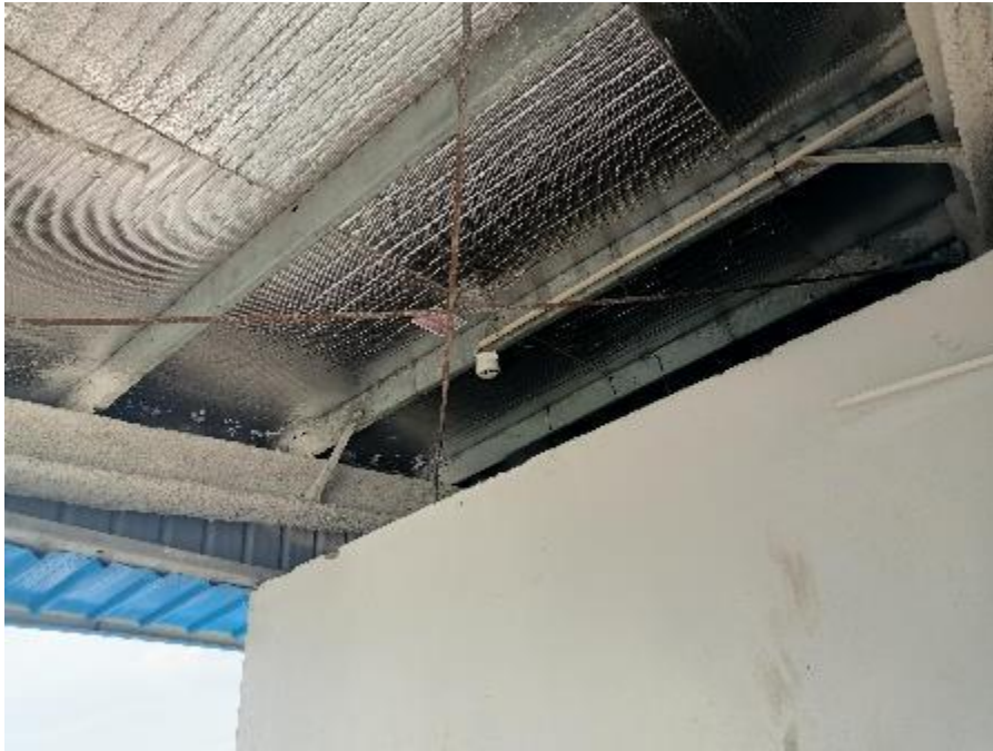
Loose cable bracing
