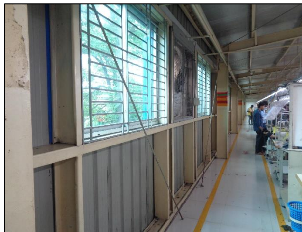
Cable bracing (1st Floor)
