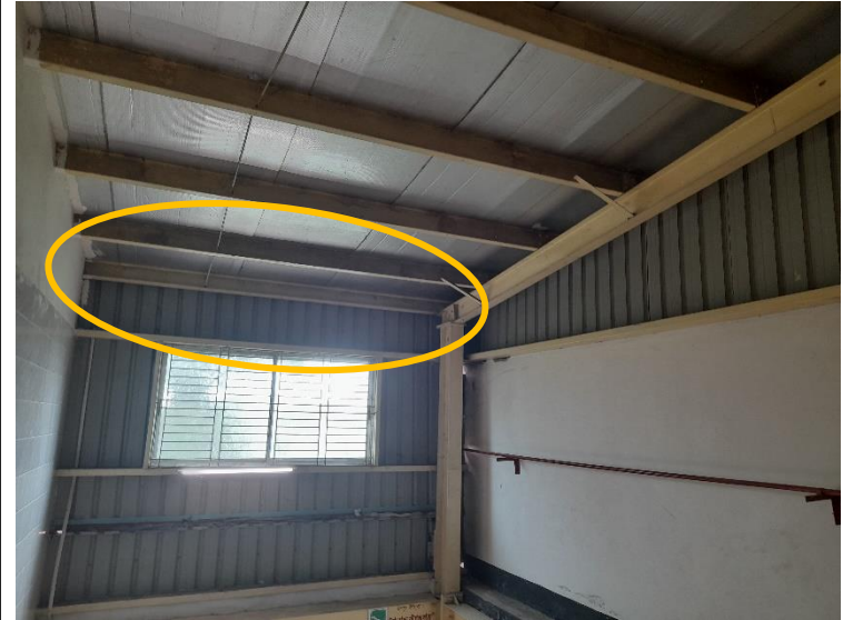
Compression strut missing in gable frame
