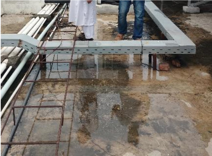
Water ponding at roof
