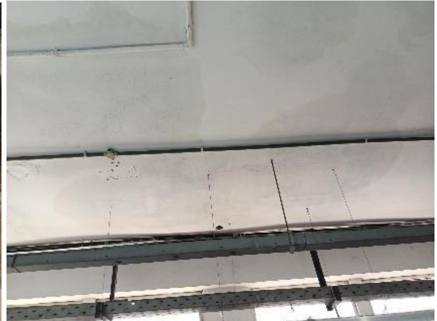
Dampness on slab soffit
