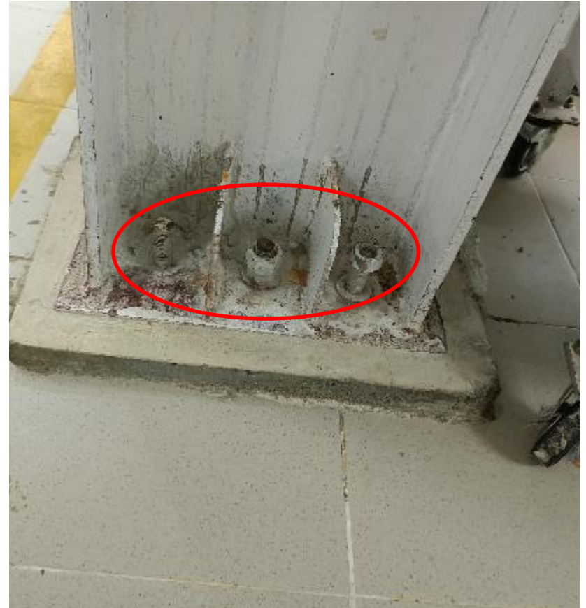
Nut missing at base plate
