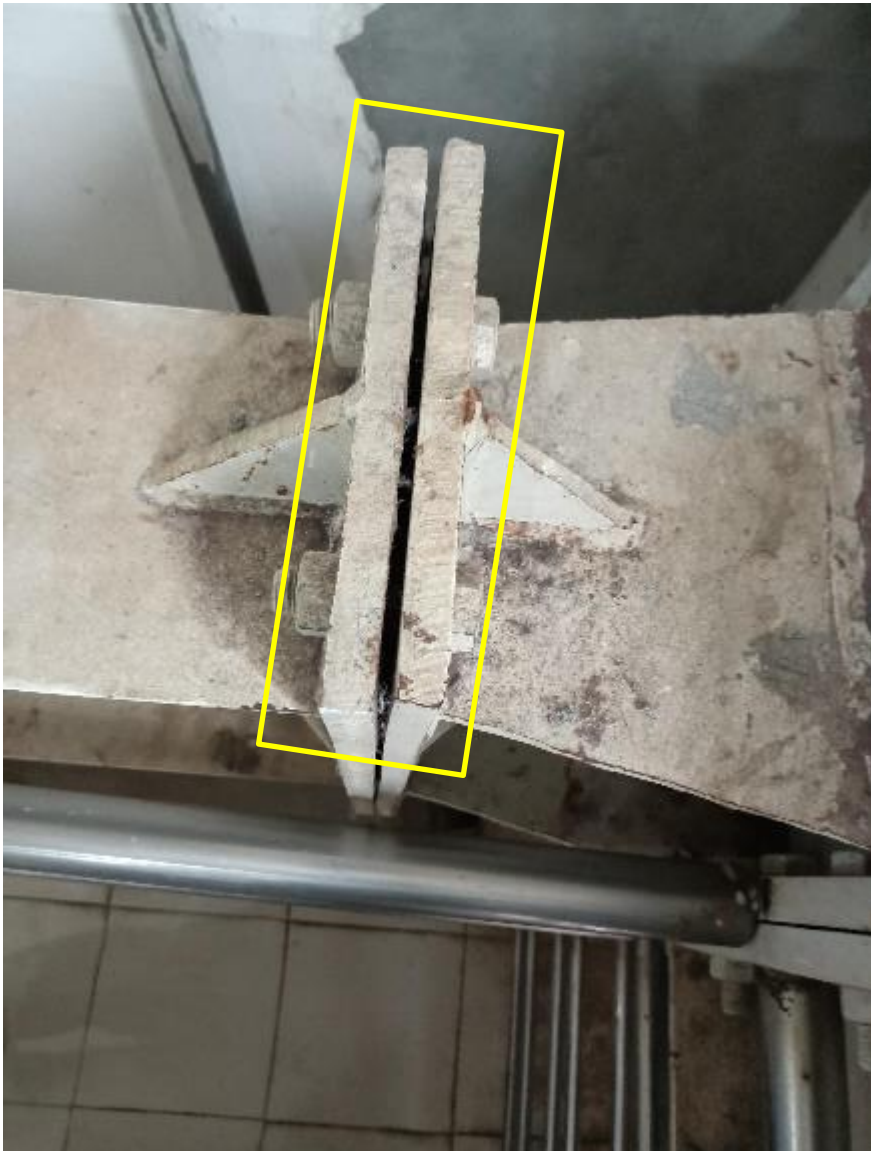
Gap observed in connections
