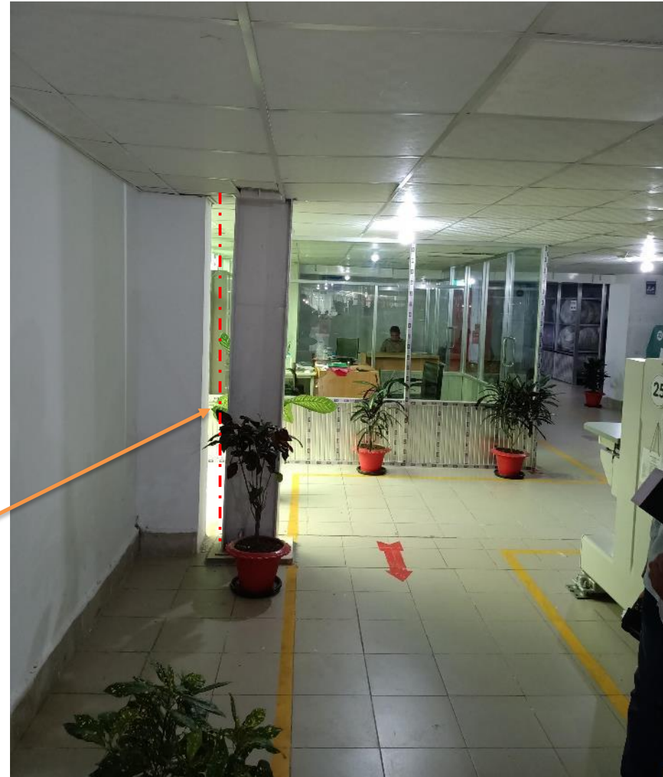
Distorted steel column
