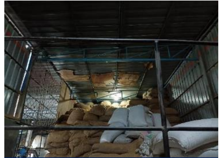
Shed-04 (Husk Boiler)
