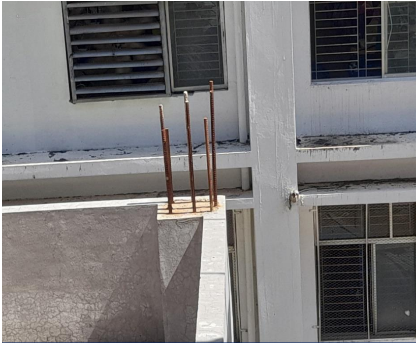
Column exposed reinforcement got rusty
