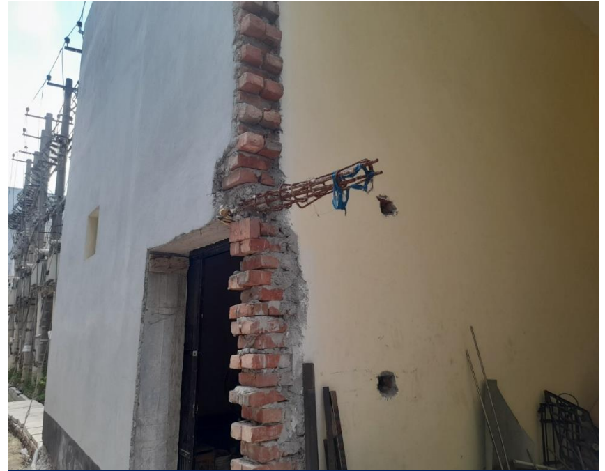
Lintel exposed reinforcement got corroded
