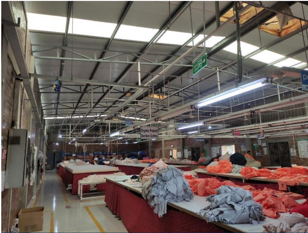
No load transfer media & bracings at roof
