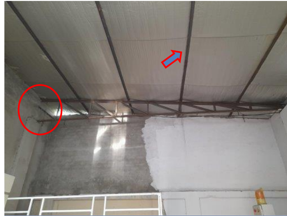
Apparently inadequate member and connection
