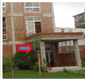
Column of porch not align with main building column grid. But drawing shown along the same column grid of main building.
