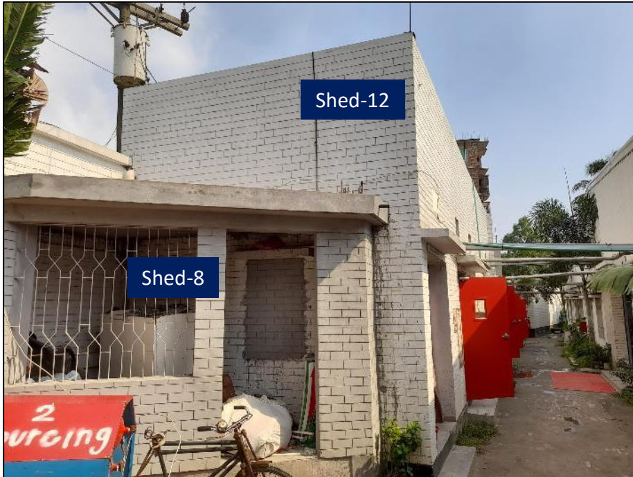
Apparently non-engineered structure with inadequate member and connection
