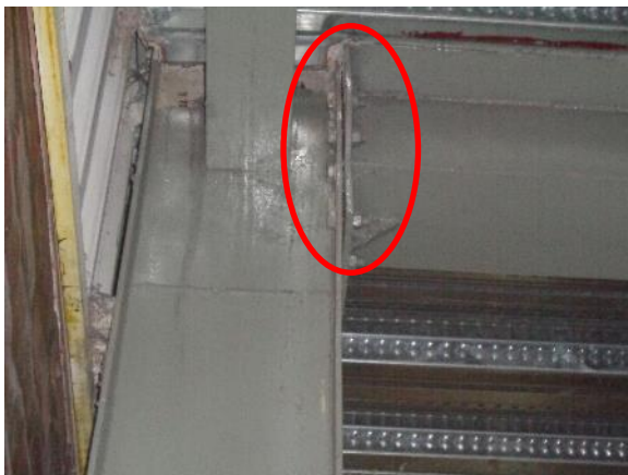
Large gap between end plates
