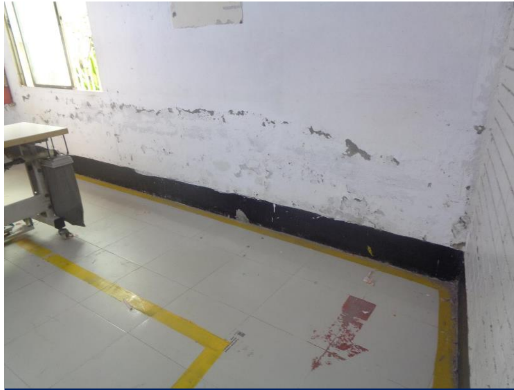
Dampness on brick wall
