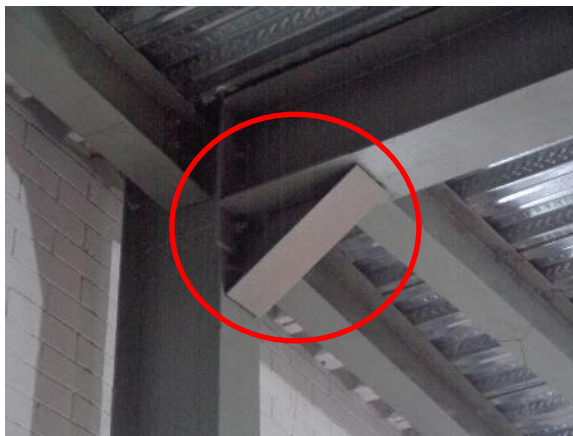
Haunch ends not connected to beam & column flanges
