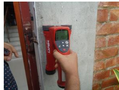
Column rebar: 4 numbers instead of 8
