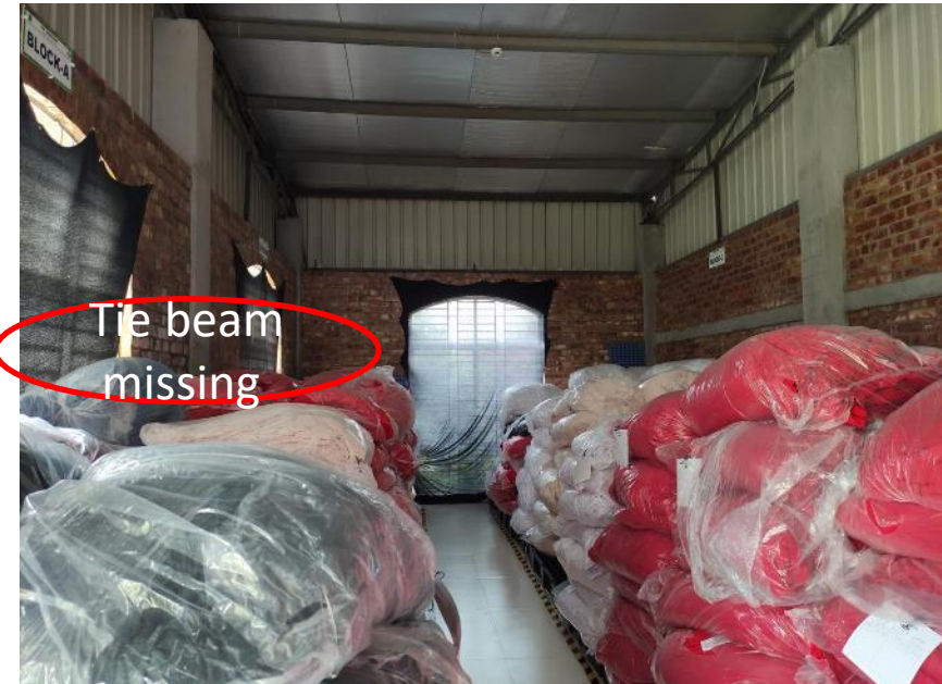
Tie Beam missing (on-site condition)
