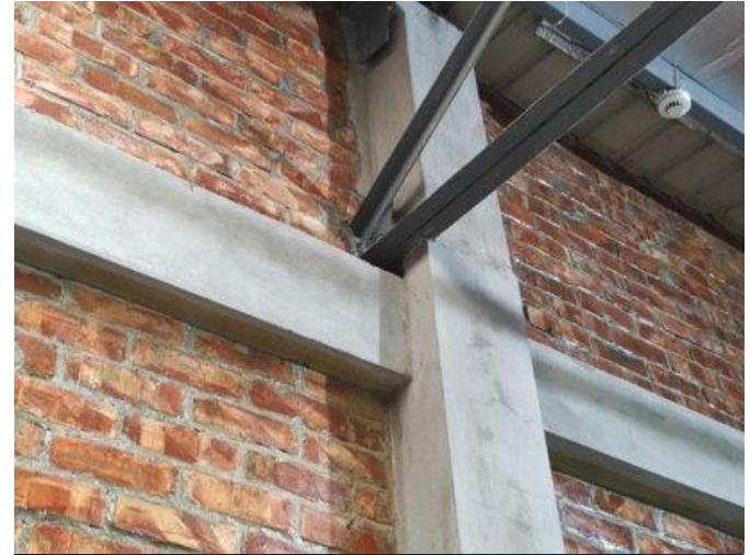
Improper connection between RC column and steel roof truss
