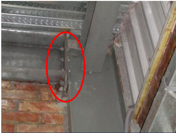
Large gap between end plates
