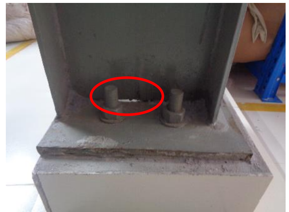
Gap between web & baseplate
