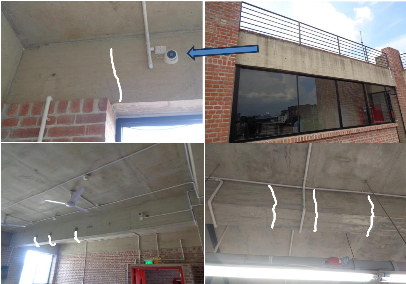
Cracks on beam in several location of all floors
