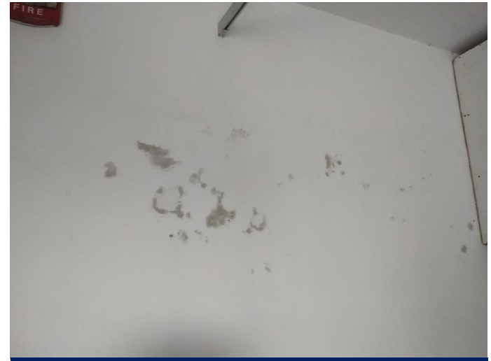
Dampness on brick wall
