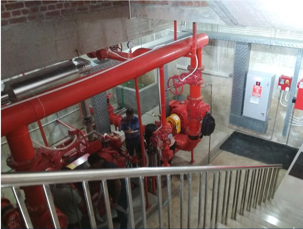
Underground fire pump room
