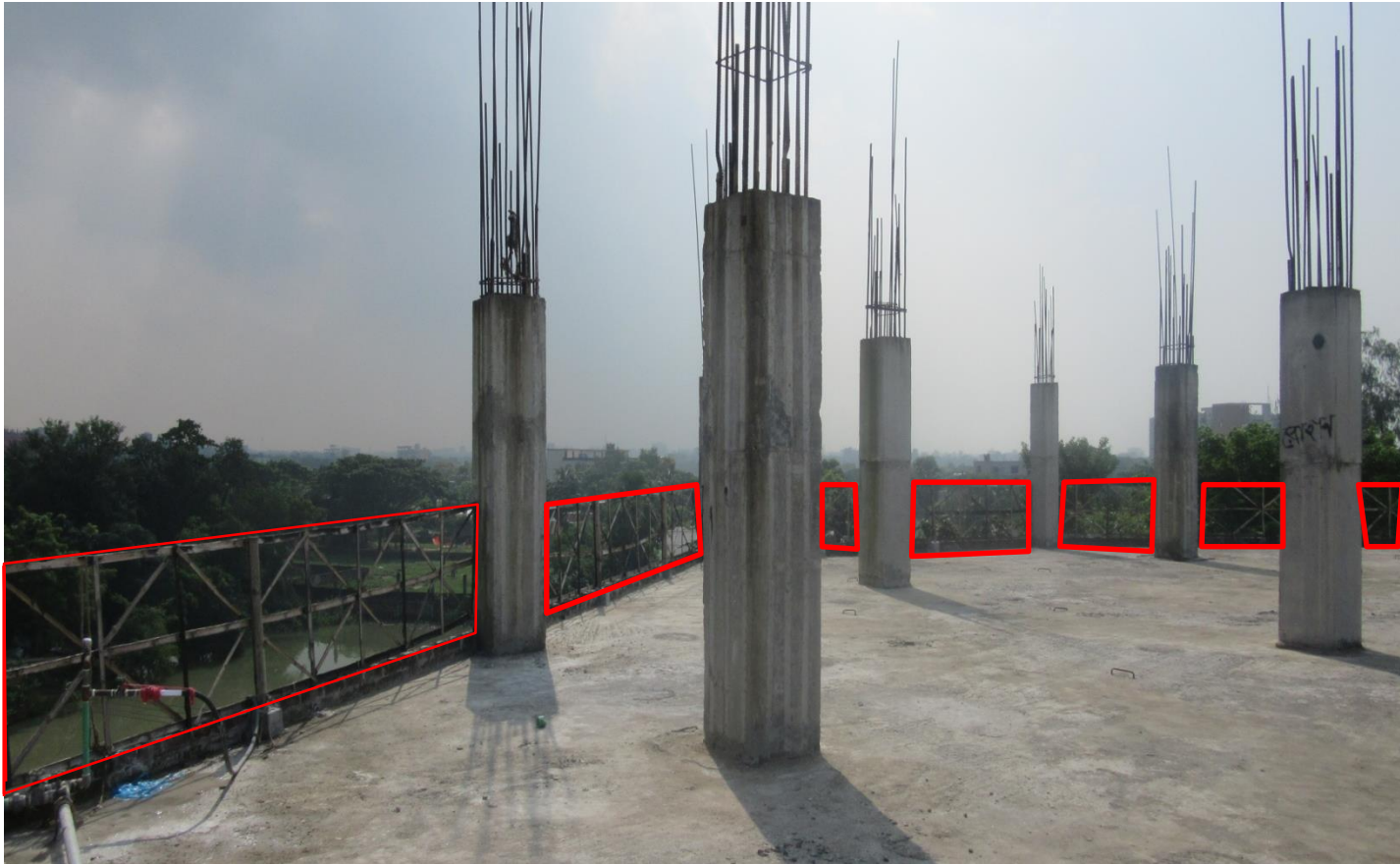
Poor edge protection on roof slab creating a safety issue
