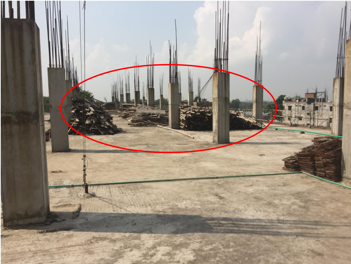
Uncontrolled material storage
