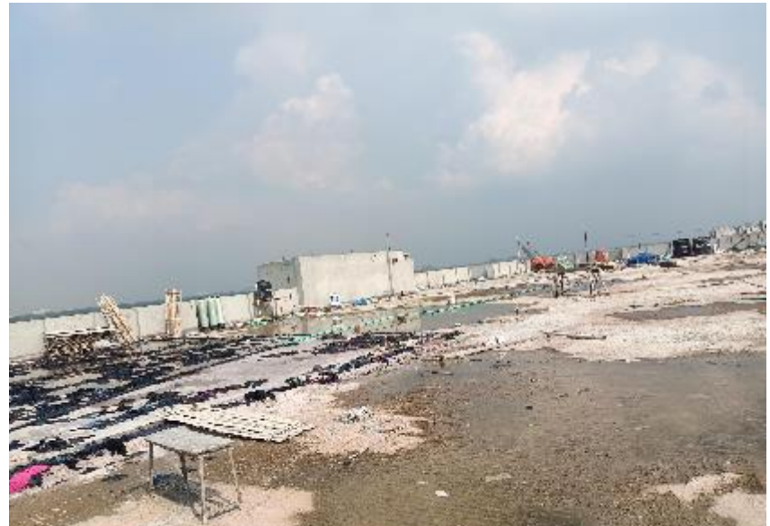
Incomplete water proofing work
