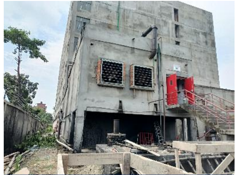
Fire Pump and Boiler Room
