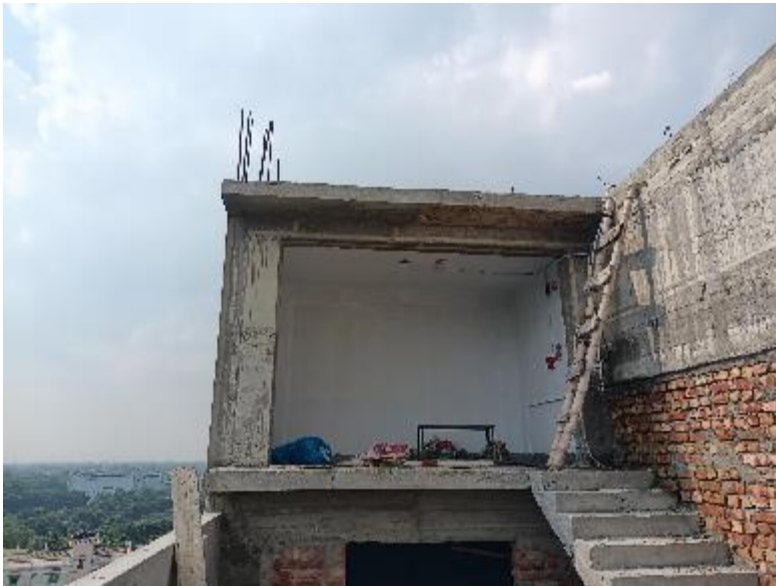
Exposed rebar at roof top column
