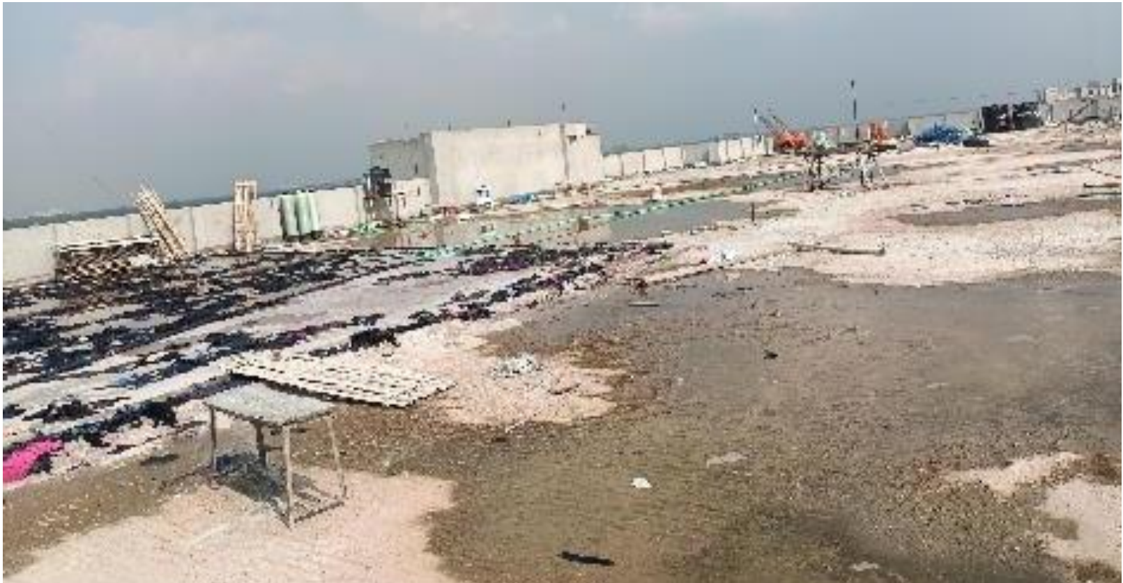
Wastage on the roof
