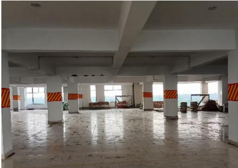
Falling hazard risk at East side windows
