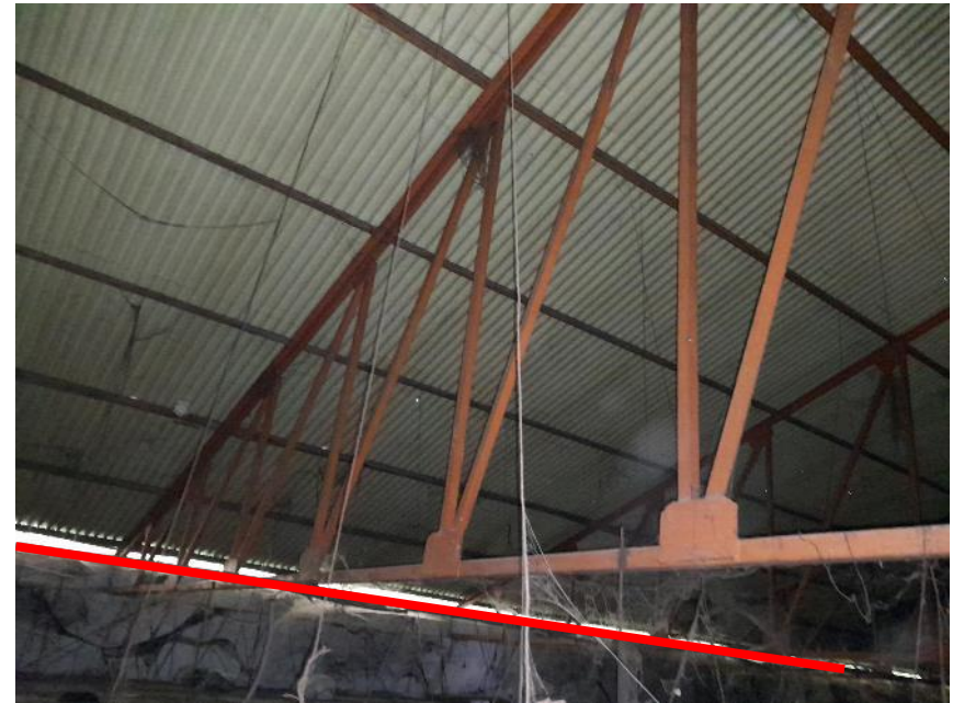
Truss tie in long direction L 50X50X6 is appeared to slender considering the length 3.66 m.
