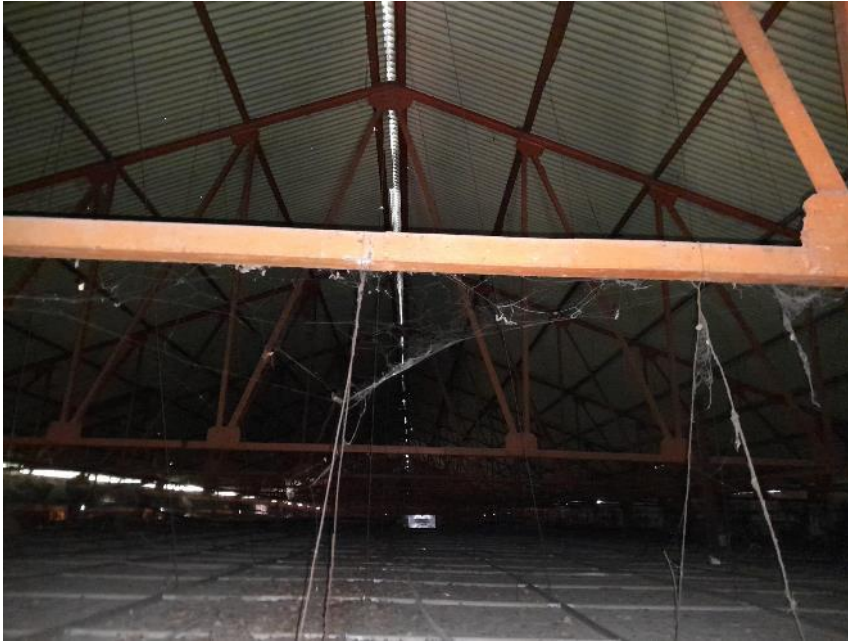
Tie member missing in mid span
