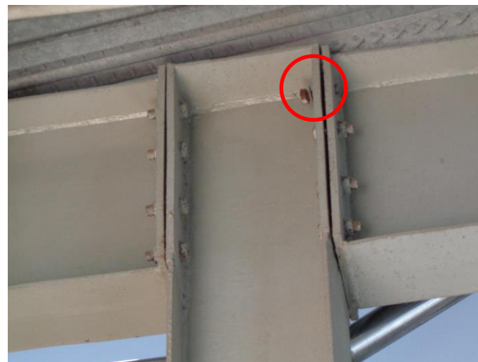
Gap between connection plates & loose bolt
