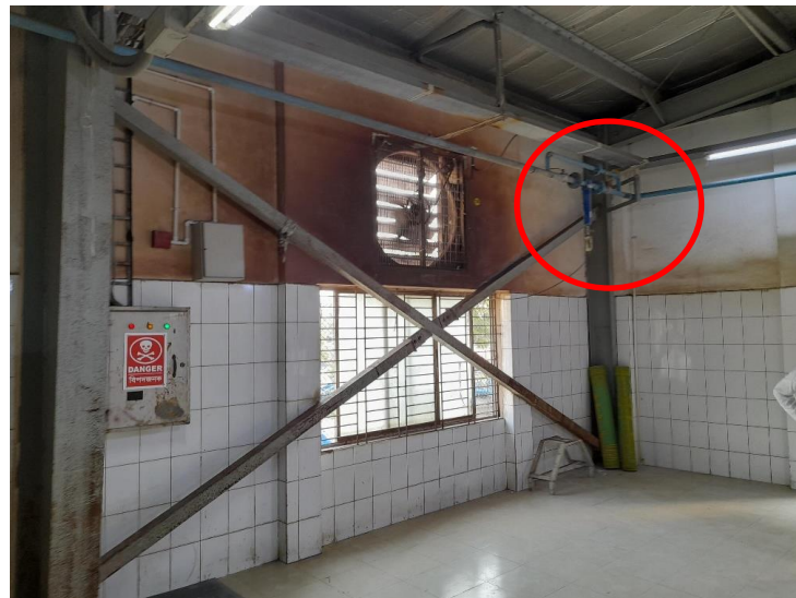
Apparently inadequate bracing gusset plate and eccentricity in joint
