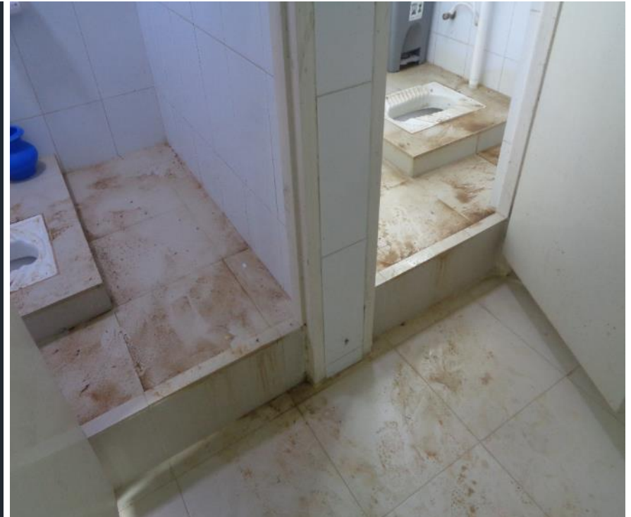
200mm build up found at toilet area
