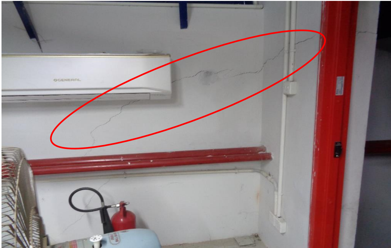
Diagonal crack was found on brick wall of mezzanine floor
