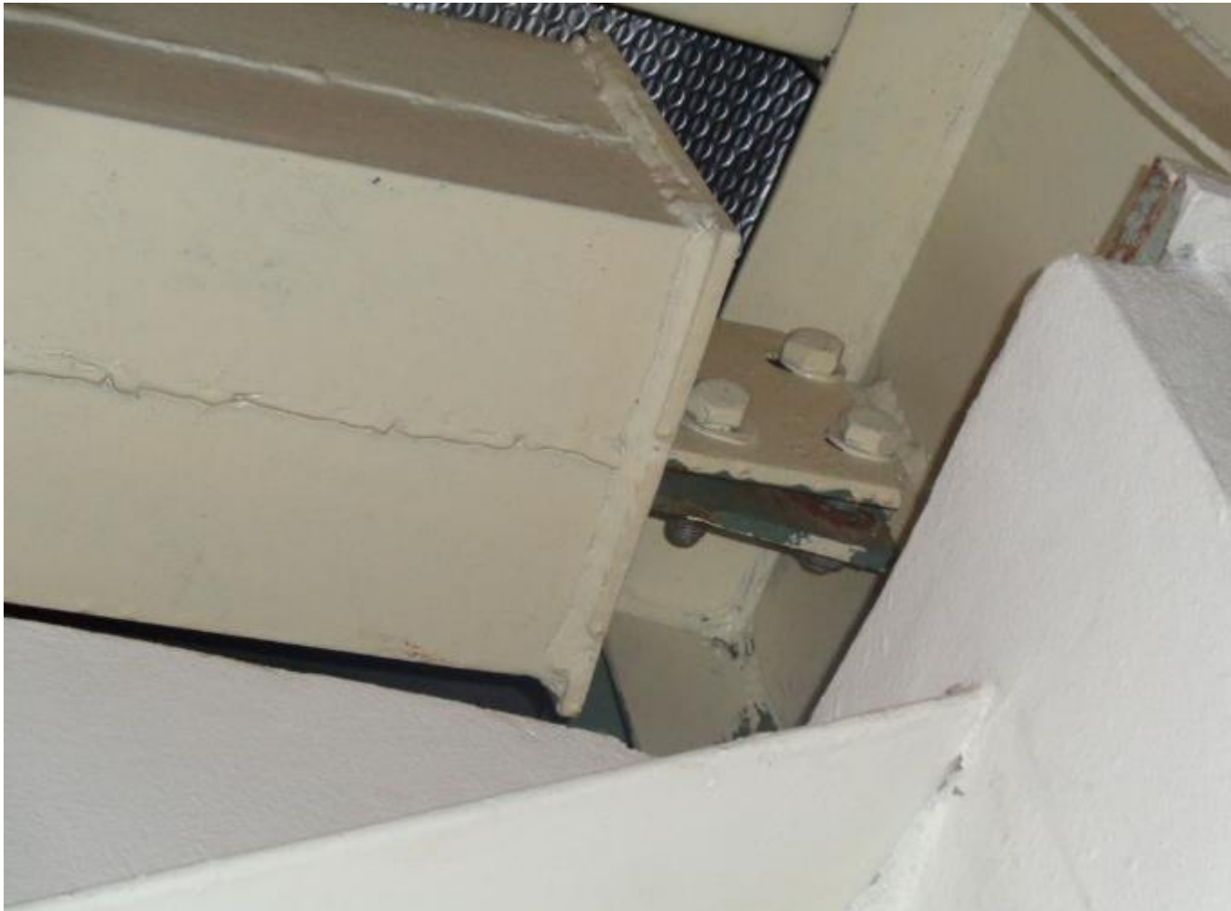
Gap observed in connections
