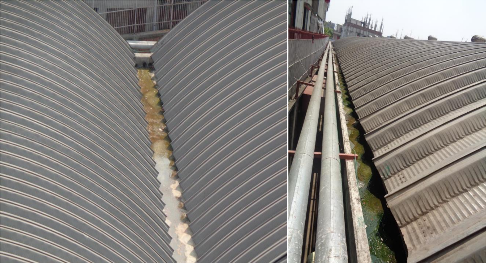
Water ponding on the concrete valley gutters of roof
