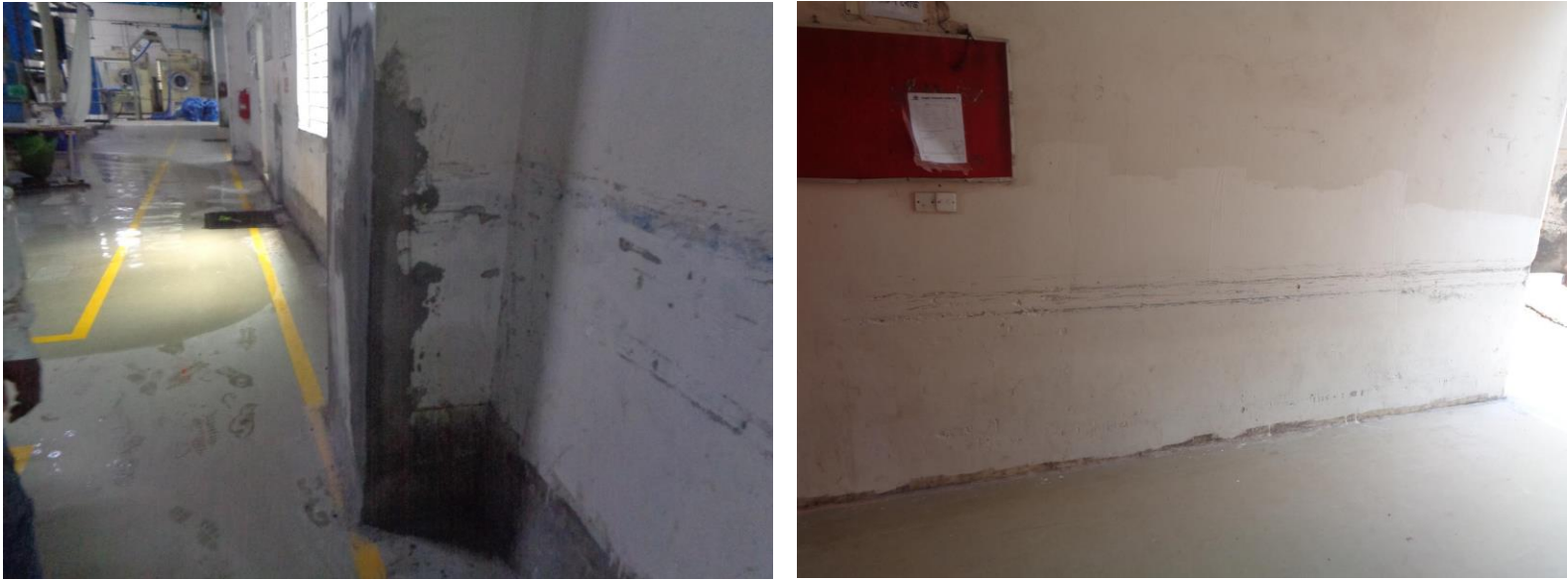
Sign of trolley impact on column and wall
