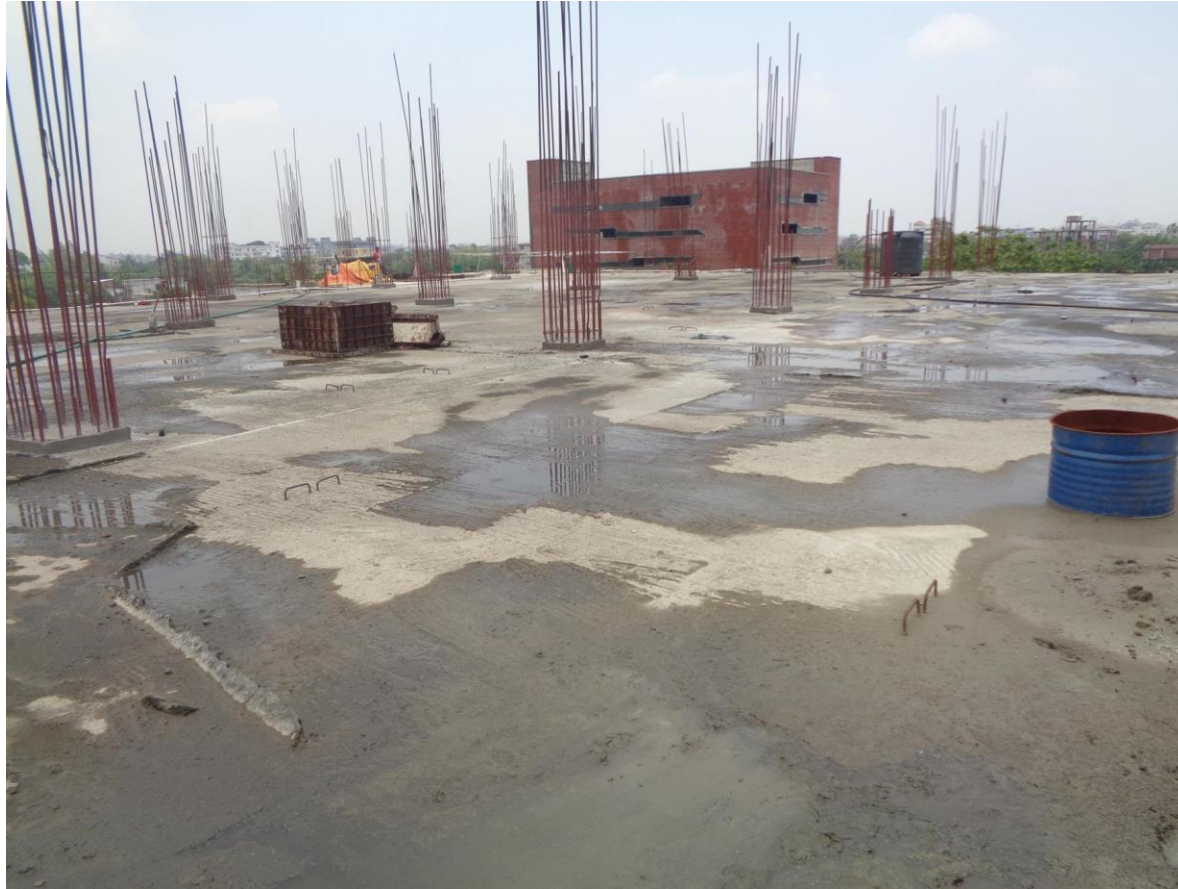
Water ponding on the roof
