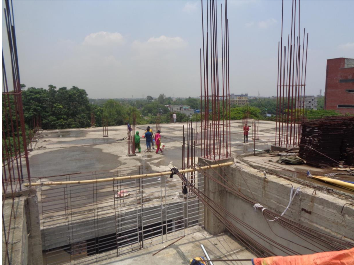
Water ponding on the roof
