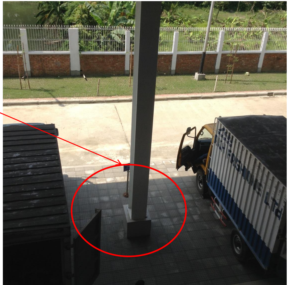
Loading bay column not protected from traffic collision
