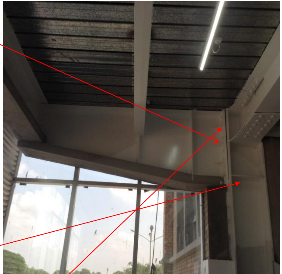
Connection of cantilevers at stair appear light
