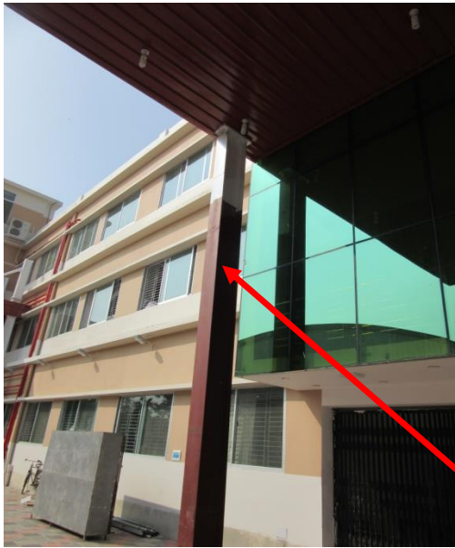
Lack of verticality of one of the Steel Columns
