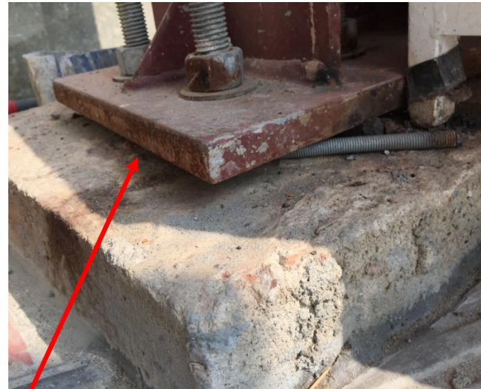
Base connection not well completed
