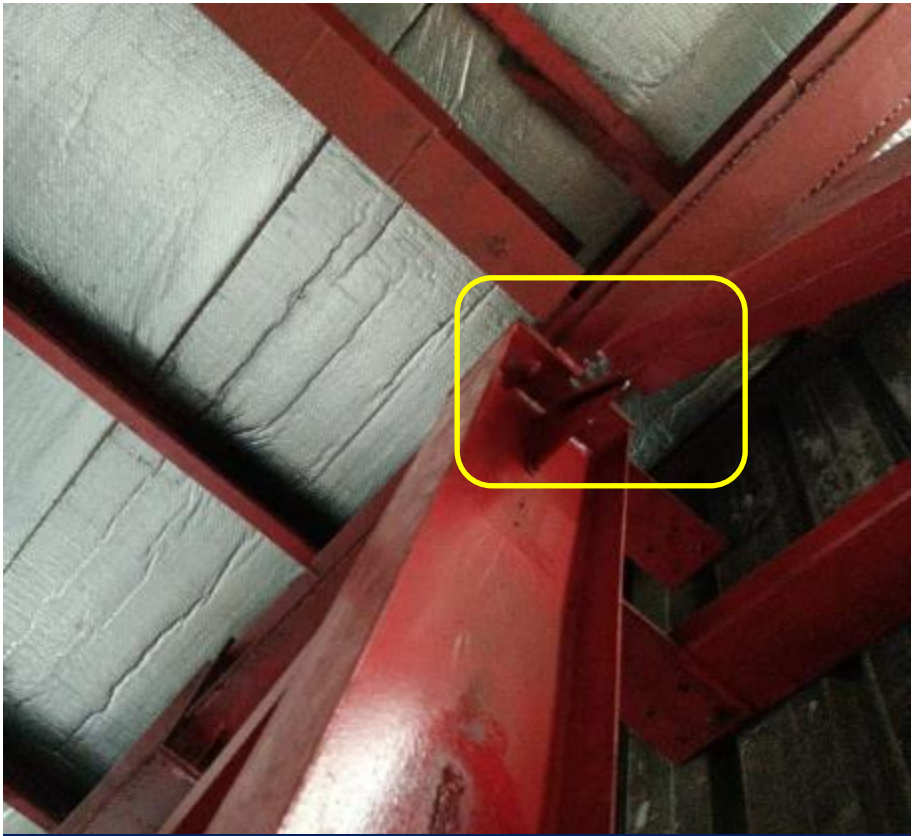
Gap observed in connections
