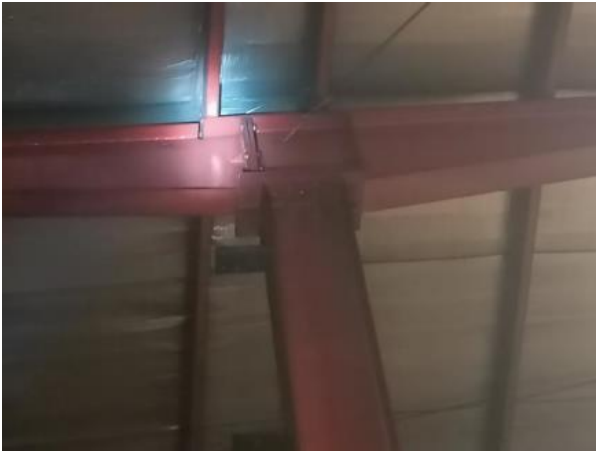
Gap observed in connections Bonded Warehouse -1
