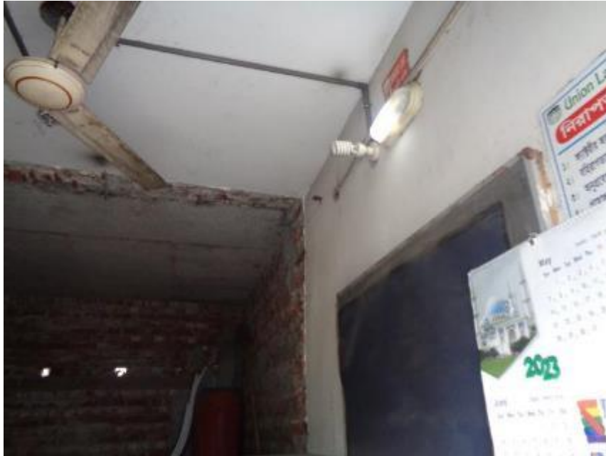
Inside of Security and Fire Pannel Room 2
