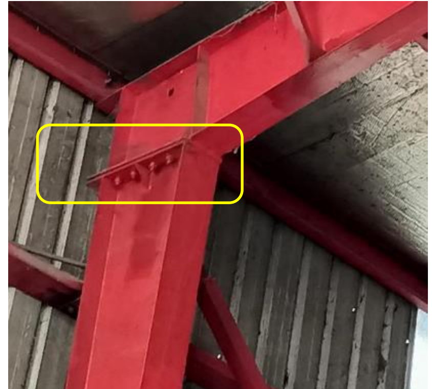
Gap observed in connections
