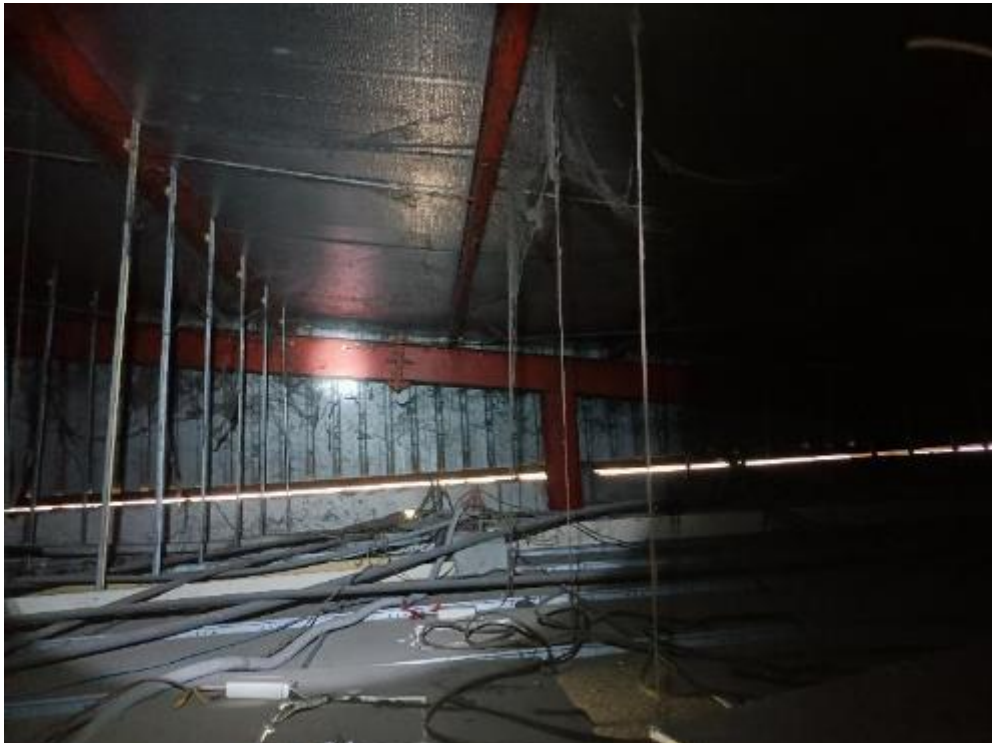
Rafter without flange bracing
