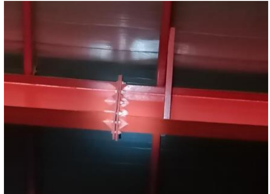
Gap observed in connections Bonded Warehouse -2
