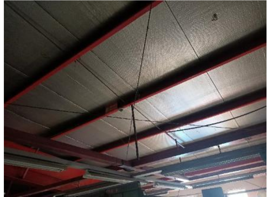
Loose cable bracing
