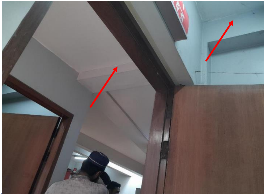
Level difference in roof slab
