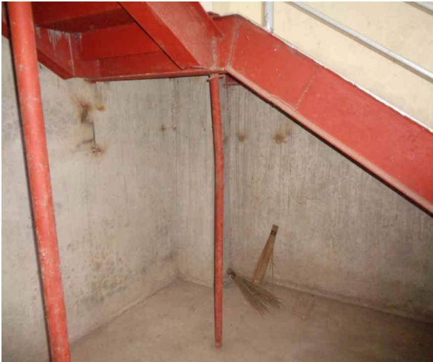
Twisted column observed under stair at basement
