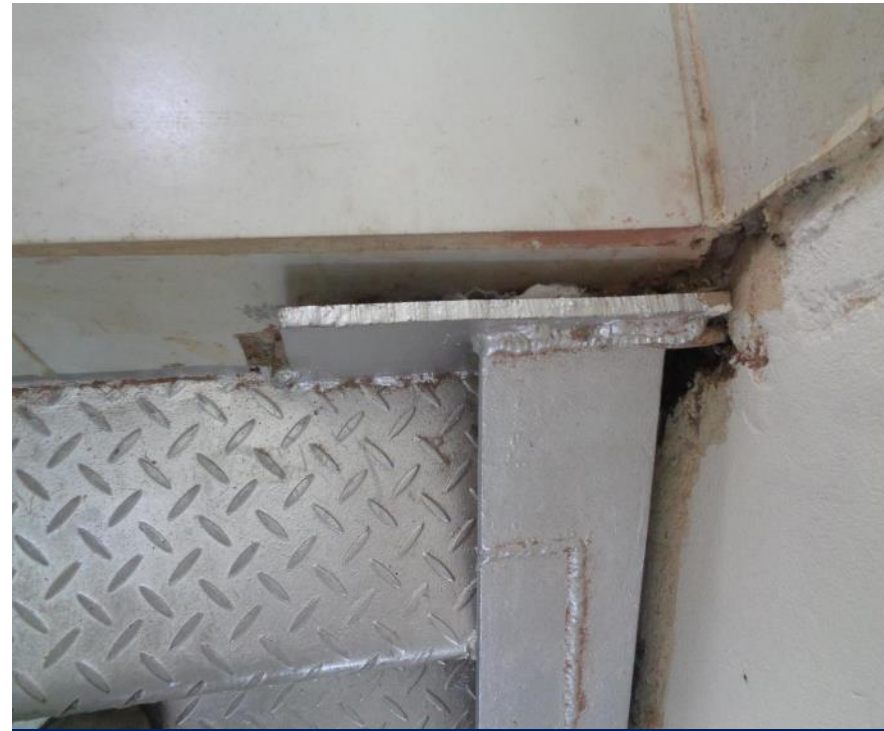
Connection gap found between steel joints
