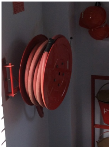
Fire Hose reel
