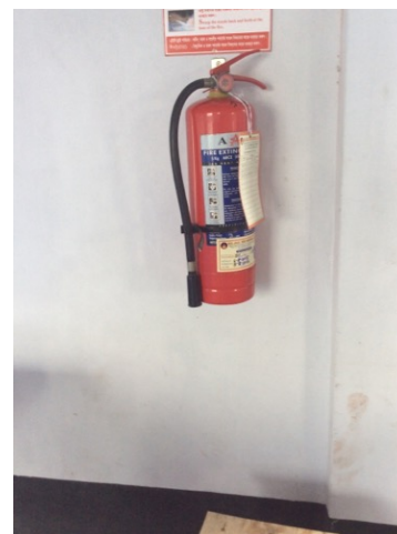
Dry chemical portable fire extinguisher
