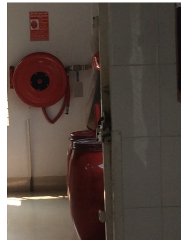
Fire Hose Reel
