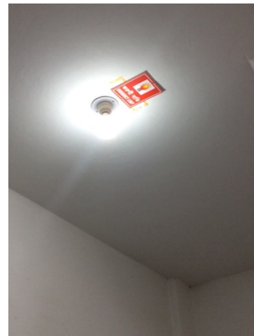
IPS Powered emergency lighting
