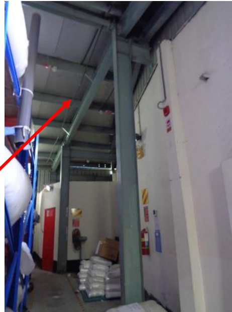
Irregular column and beam
