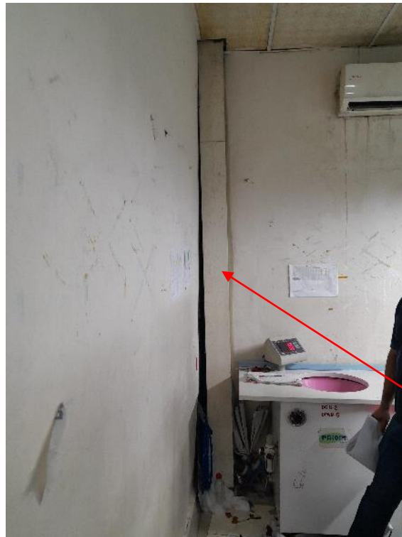
Steel column out of plumb
