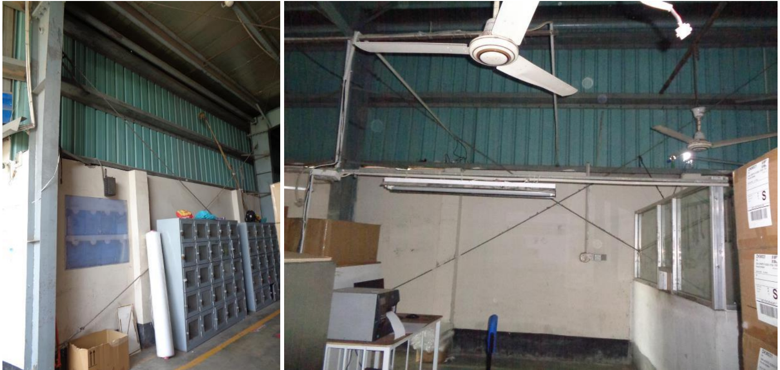
Loose cable bracing at wall and roof
