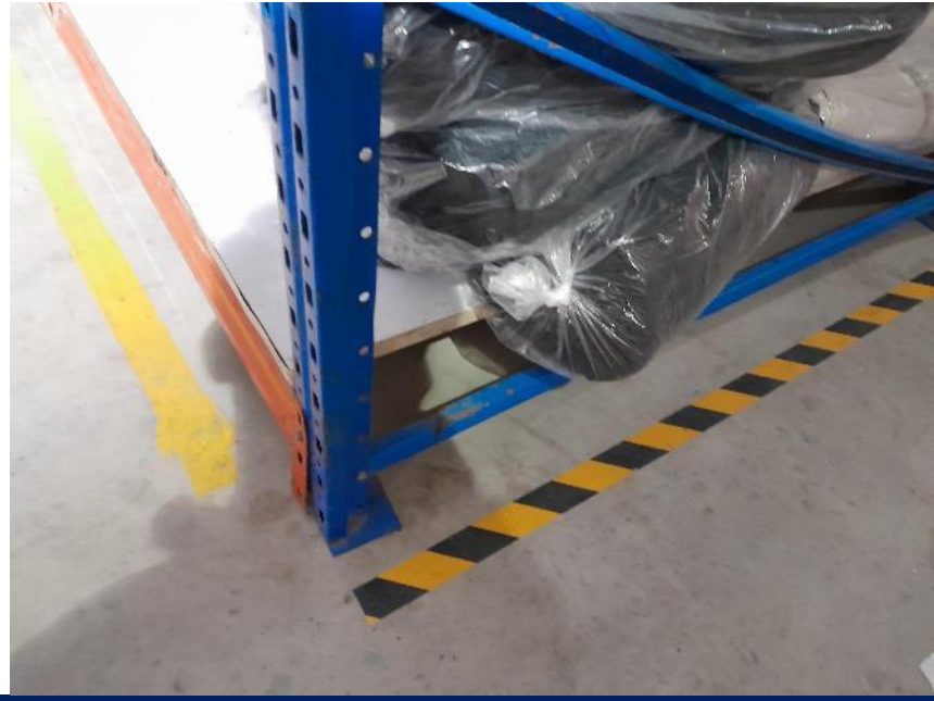
Steel racks without anchored/braced.
