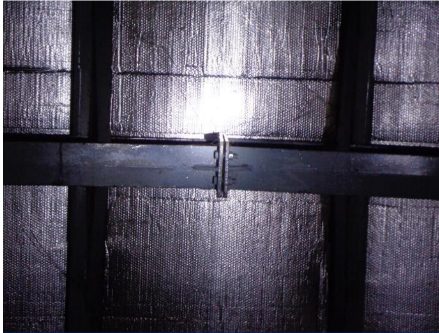
Onsite connection gap (Finished goods Warehouse)
